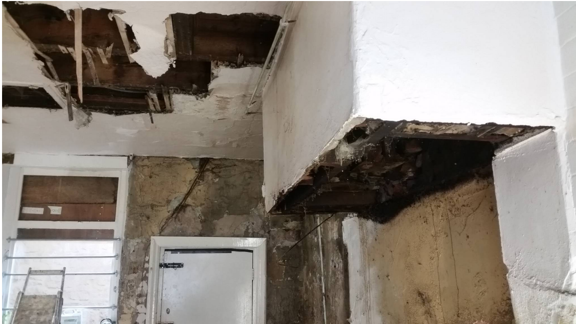
Picture 5: The room of the proposed seating area has incomplete plaster board. This accounted for its low sound insulation of DnT'W + C (c;ctr) 39 (-2,-7) \text{ dB} .
