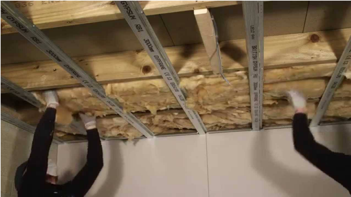
Picture 6: Resilient bar ceiling. In the recommended design below, the original joists are insulated and the resilient bar is fixed on hangers as opposed to directly onto the wooden joists. Source:
