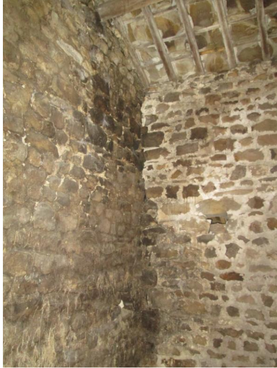
Photo 9 – Separation between Right-Hand Gable Wall and Internal Wall
