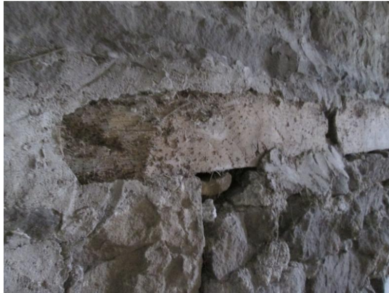
Photo 10 – Decayed Timber Lintel
