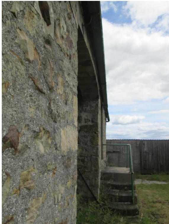
Photo 18 – Outward Bow of Arch Stonework above Main Entrance
