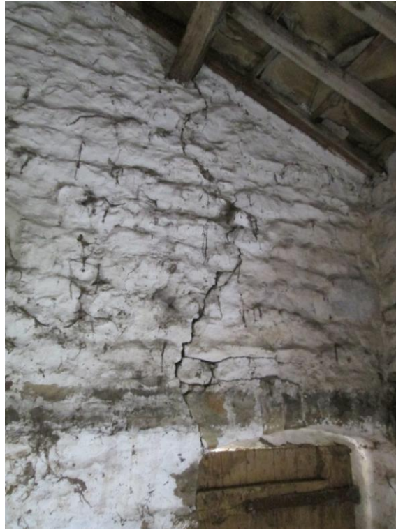
Photo 12 – Crack in Internal Face of Wall on Left-Hand Side of Entrance
