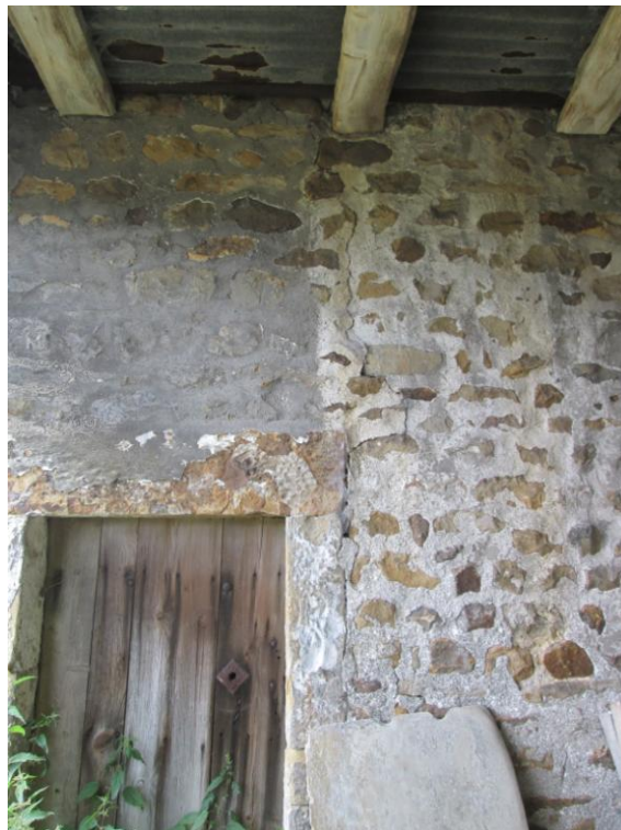
Photo 13 – Crack on External Face of Wall to Left-Hand Side of Entrance
