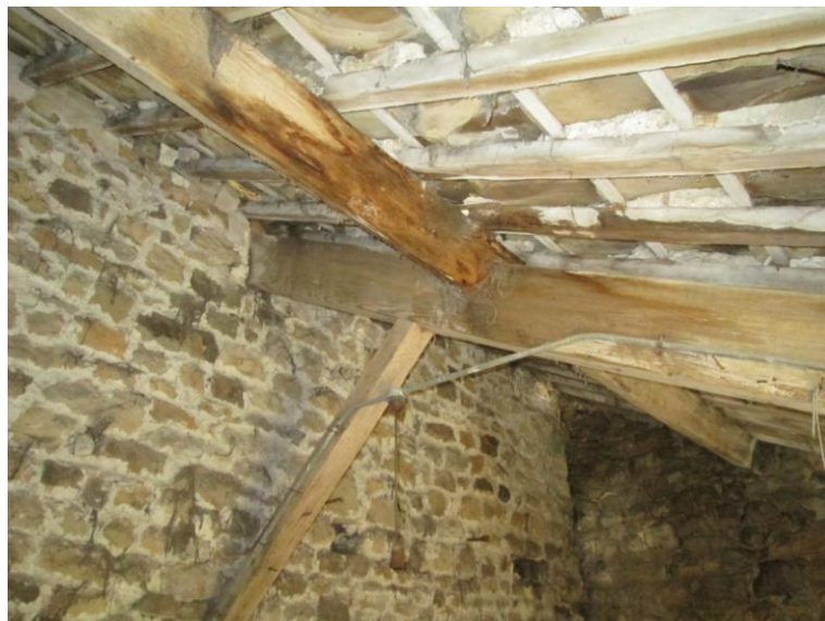
Photo 8 – Stained and Decayed Purlin over Workshop
