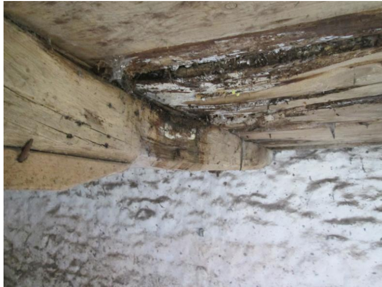
Photo 15 –View of Decayed Workshop Floor Beams
