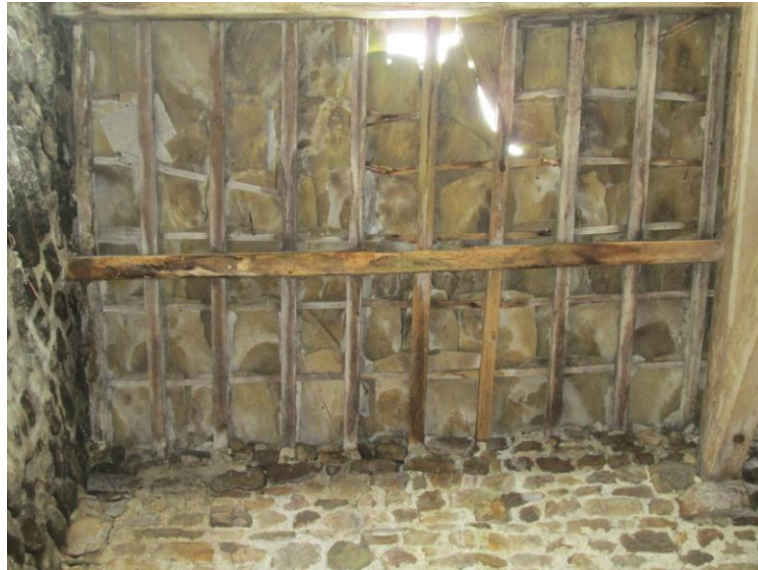
Photo 5 – Left-Hand Gable - Decayed Purlins and Rafters
