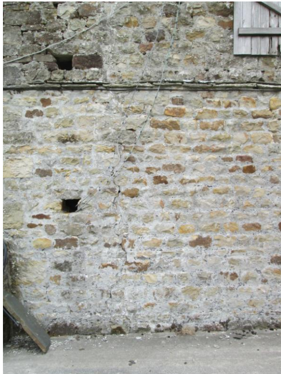
Photo 20 – Crack in Left-Hand Gable Wall (Rear)
