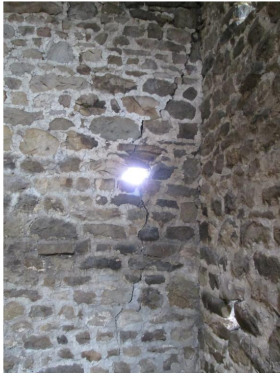
Photo 9a – Steep Diagonal Crack where Rear Wall joins Right-Hand Gable
