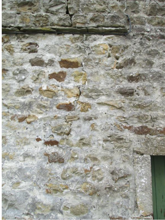
Photo 19 – Crack in Left-Hand Gable Wall (Front)
