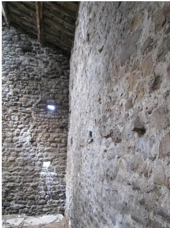
Photo 14a –Rear Wall leaning towards Shippon
