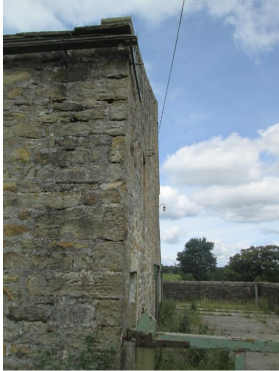
Photo 17 – Outward Curvature of Right-Hand Gable
