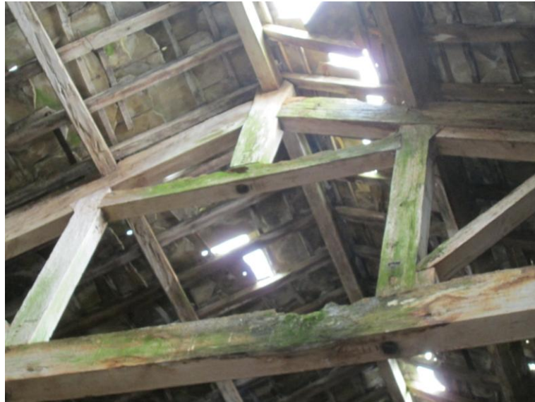
Photo 7 –Stained and Decayed Roof Truss
