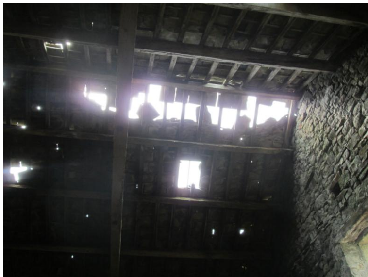
Photo 6 – Missing Slates and Damaged Timbers
