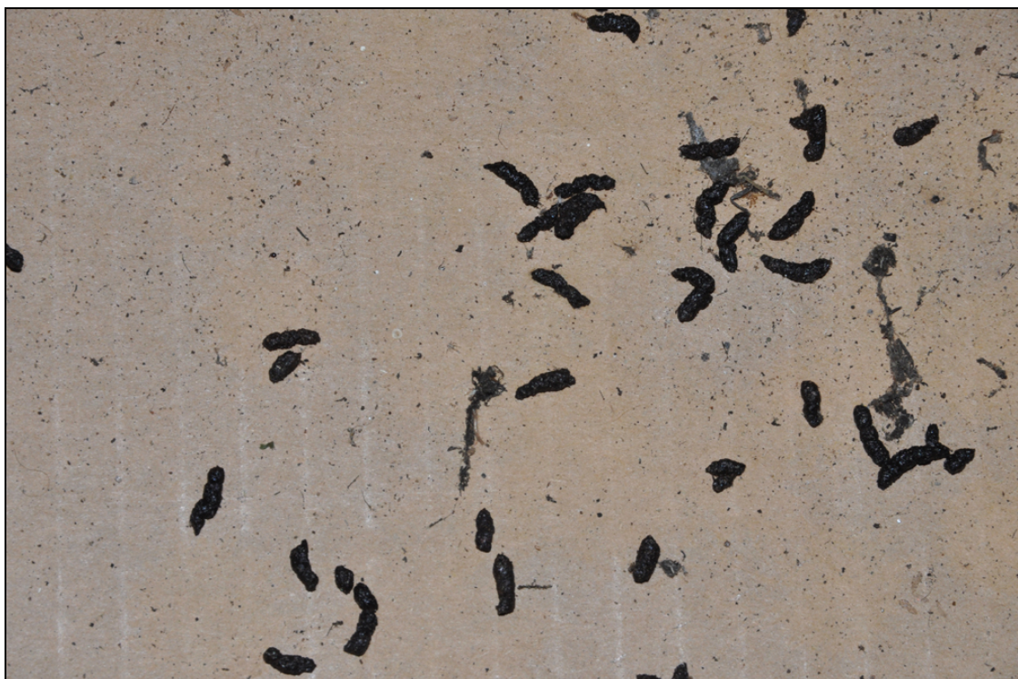
Close-up image of bat droppings on survey sheet in roof void of Garnet House. April 2017
