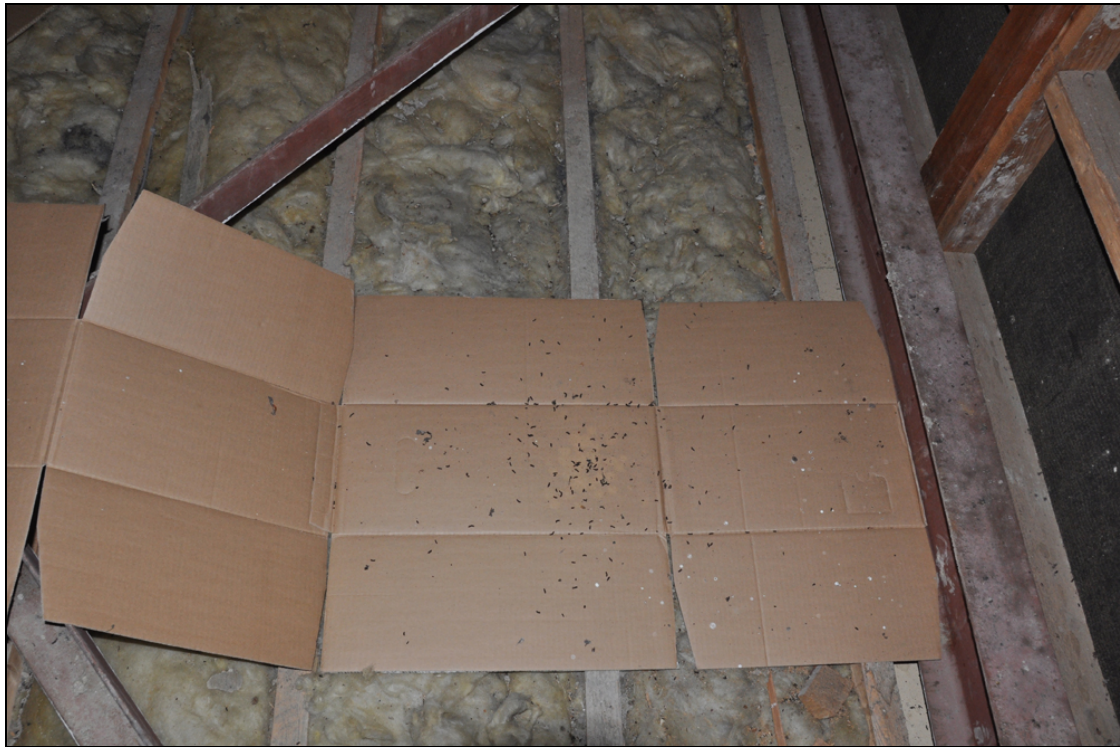
Bat droppings on survey sheet in roof void of Garnet House. April 2017
