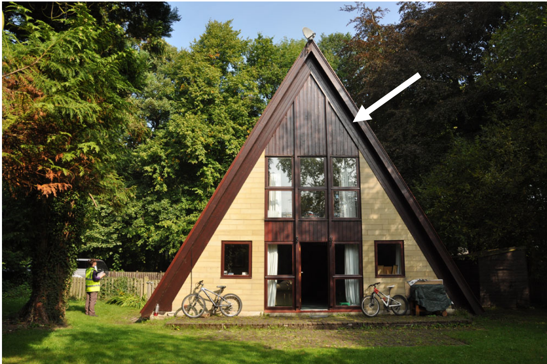
Garnet House (bat roost) – south elevation with 2014 bat exit point shown by white arrow. September 2014
