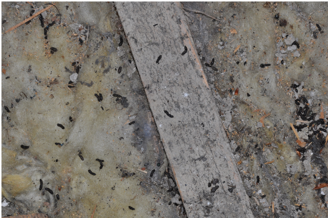
Scattered bat droppings in roof void of Garnet House. September 2014
