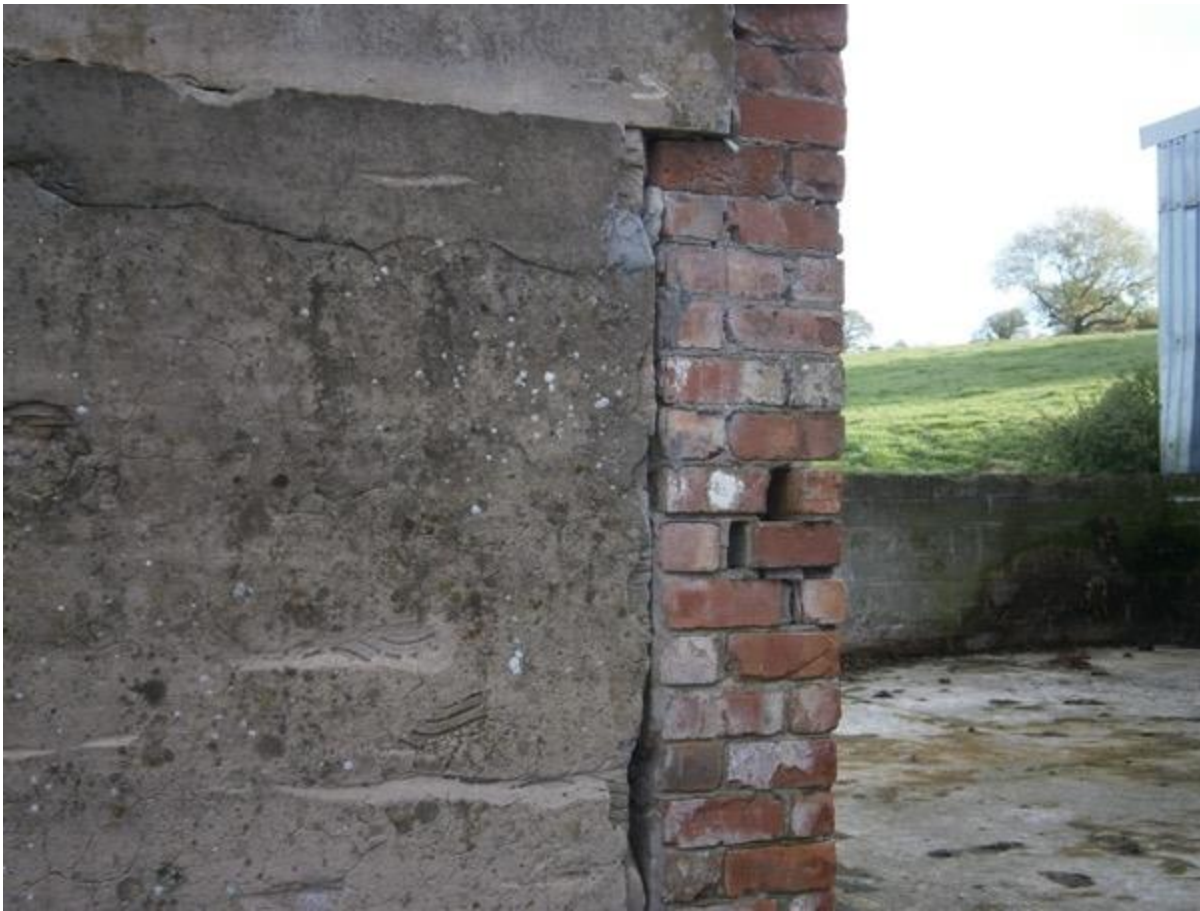
Photo 4 - South West Elevation – damaged corner
