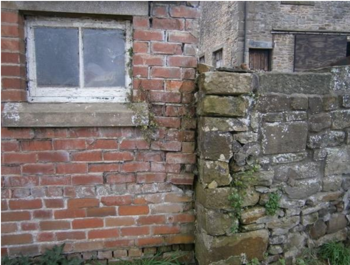
Photo 11 - North West Elevation – damage at gable corner
