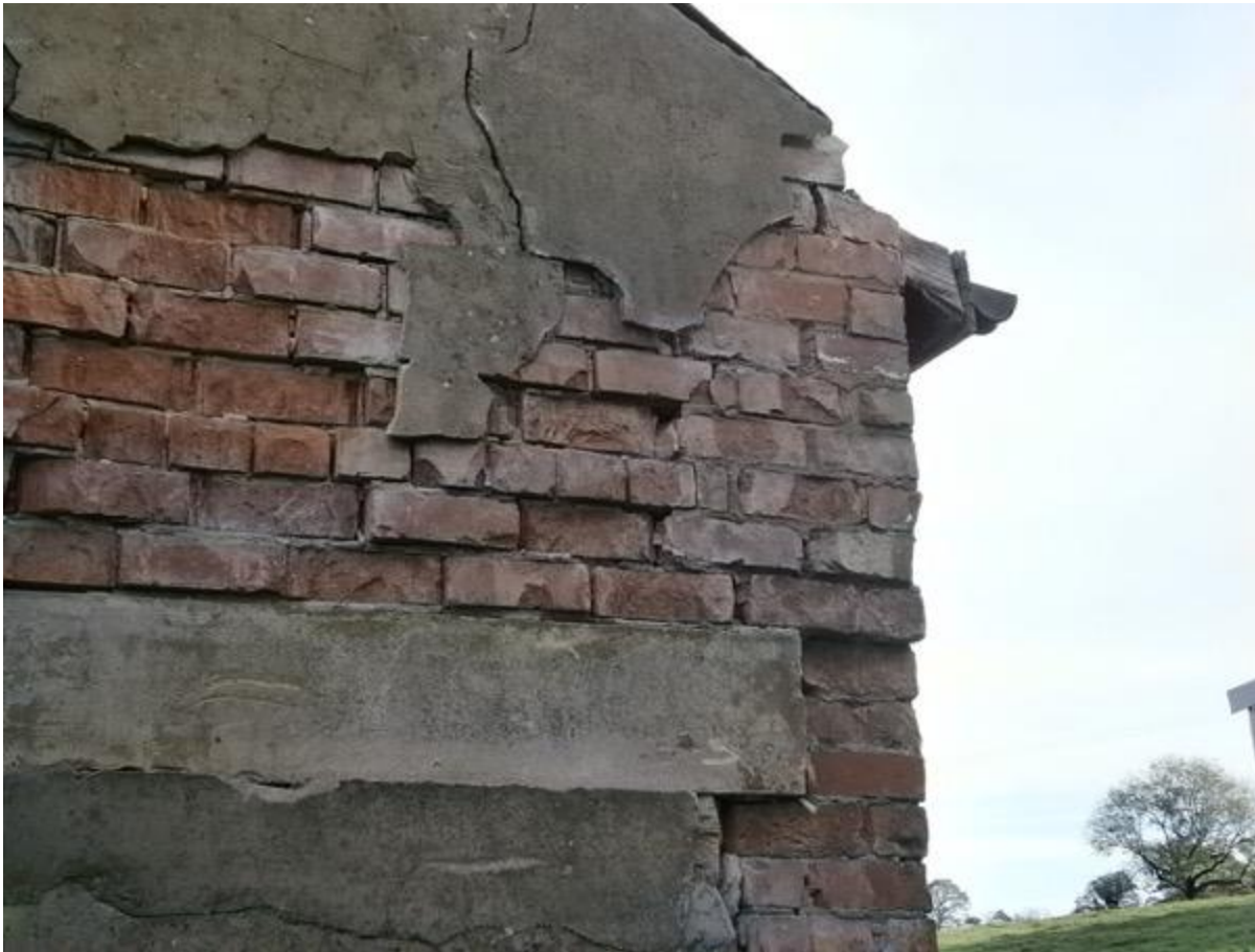
Photo 3 - South West Elevation – damaged corner
