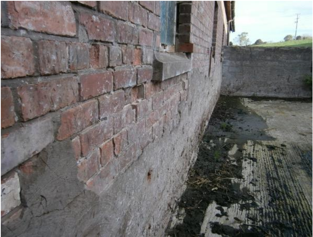
Photo 7 – South East Elevation – blown bricks
