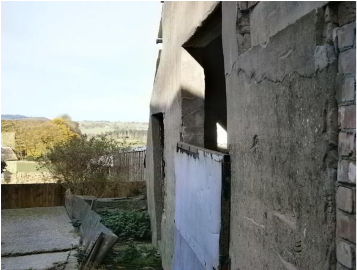
Photo 5 – South West Elevation – showing bowing/movement
