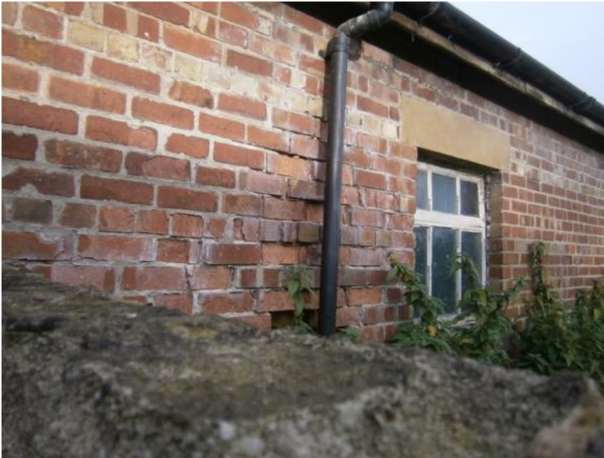
Photo 9 – South East Elevation – damaged around downspout
