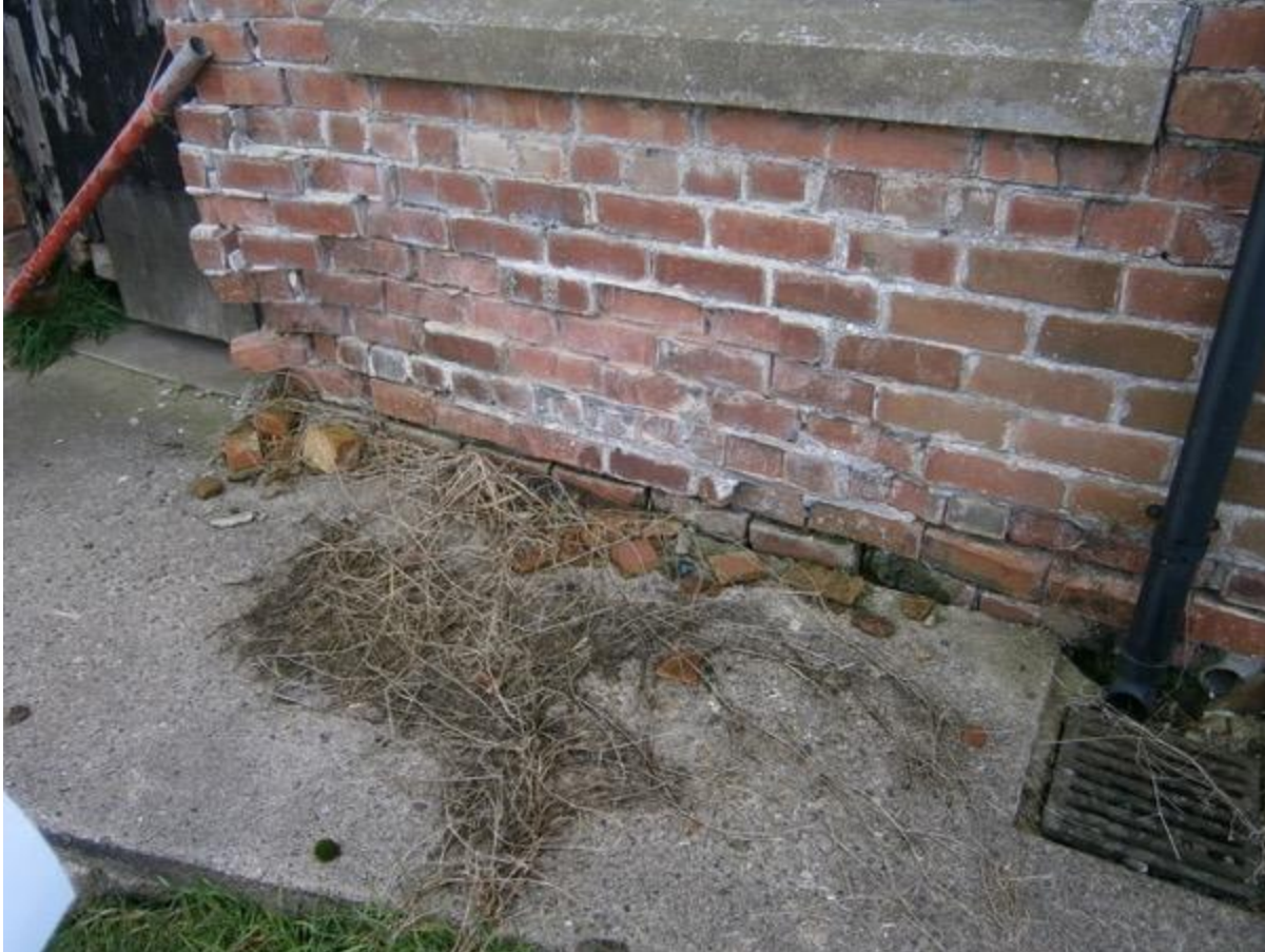
Photo 12 - North West Elevation – damage at below window
