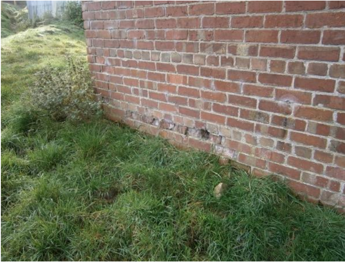
Photo 16 - North East Elevation – row of damaged/blown bricks
