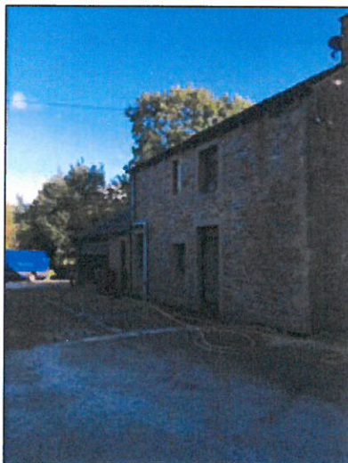
Image 6 : North elevation. This photo also shows access between the cottage and farm
