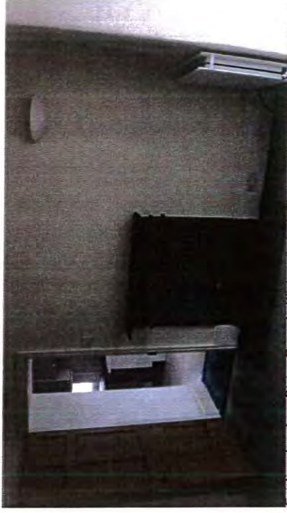
Poorly fitting sash window in front Bedroom, with vegetation ingress.
