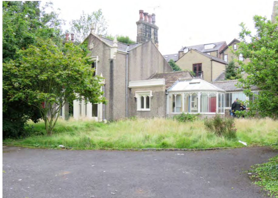
View towards front (East) elevation from tarmac parking area, showing overgrown gardens.
