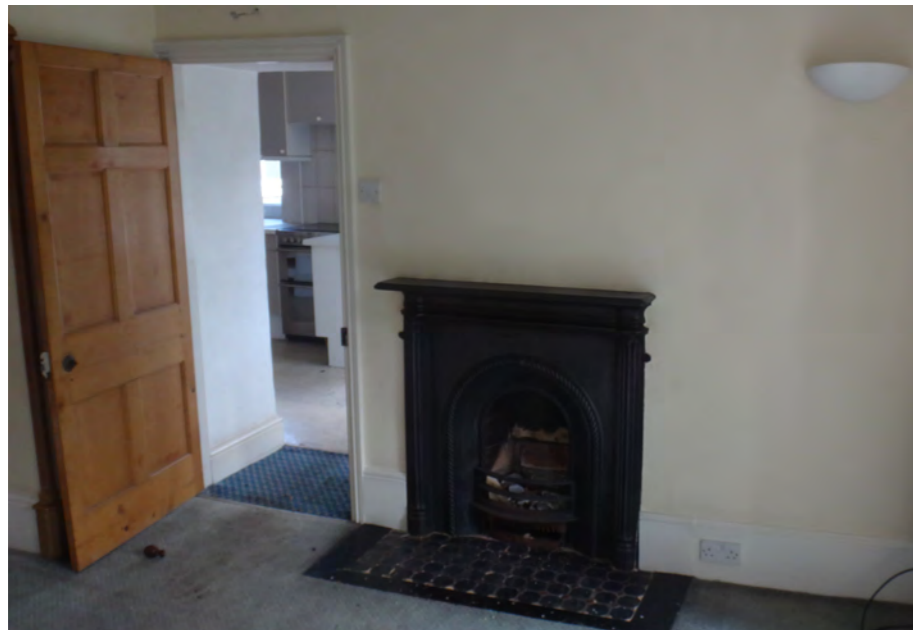
Existing door from Dining Room to Kitchen (to be infilled on Kitchen side, with recess or cupboard retained on Dining Room side).
