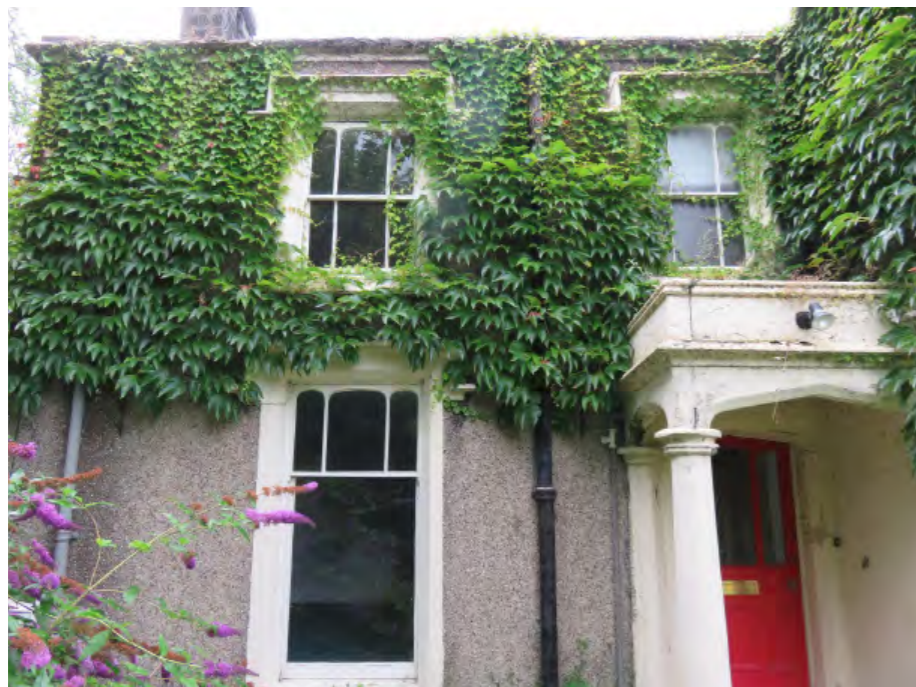
Overgrown ivy on East elevation and entrance porch.
