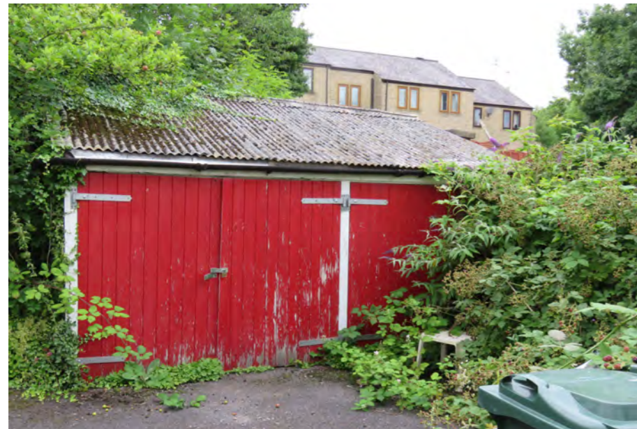
Overgrown detached double garage adjacent to North boundary.
