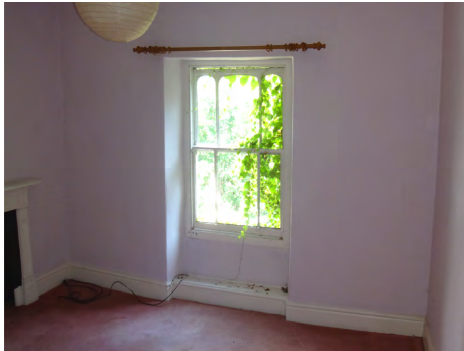
Poorly fitting sash window in front Bedroom, with vegetation ingress.
