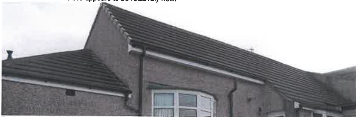
The rear roof pitch being affected by the development .
