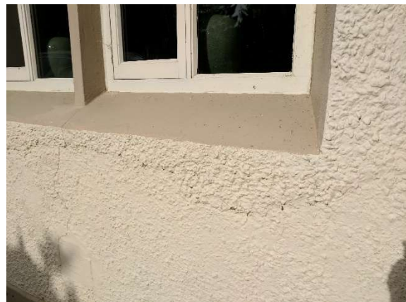
Figure 1 - Patched render, highlighting previous repairs
