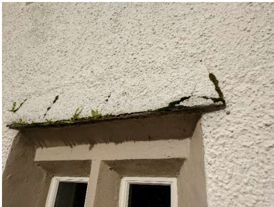
Figure 2 - Moss growing in cracks of render, allow water to sit in the cracks and penetrate further in to the fabric of the building
