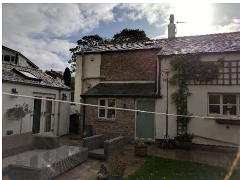
Figure 3 - Areas where render has fallen off previously, then cleansed off by applicant until Planning Application has been submitted
