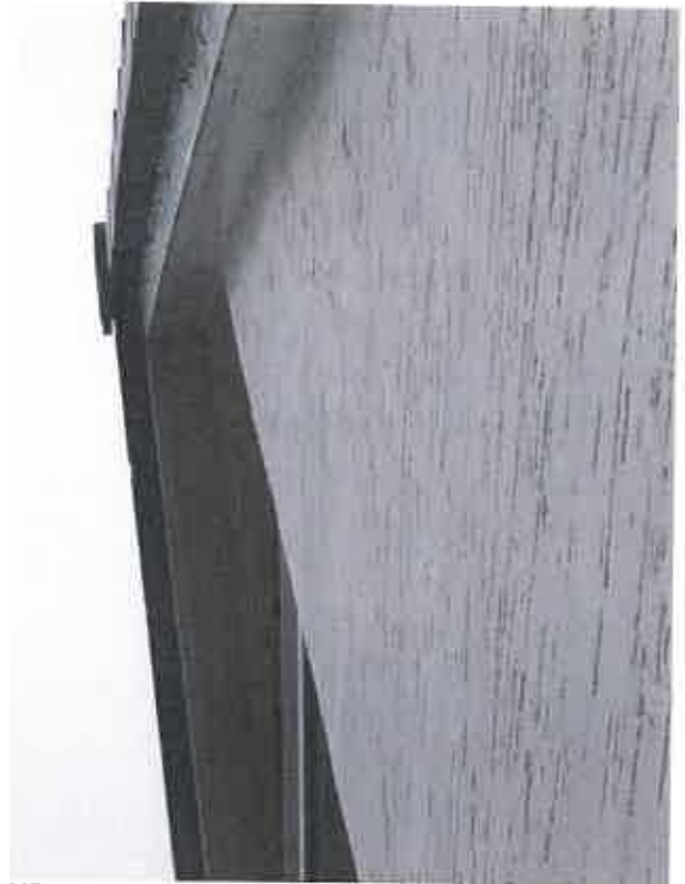
NE front elevation with tight fitting soffits.
