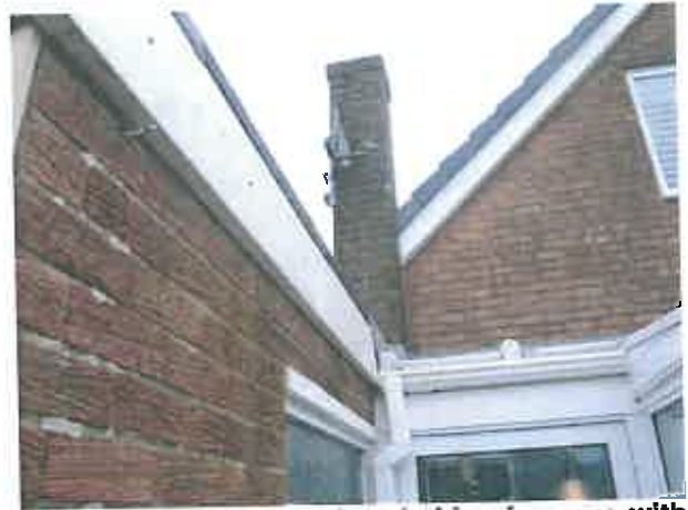
SW rear elevation (part) and side of garage with tight fitting fascia boards (no gaps)
