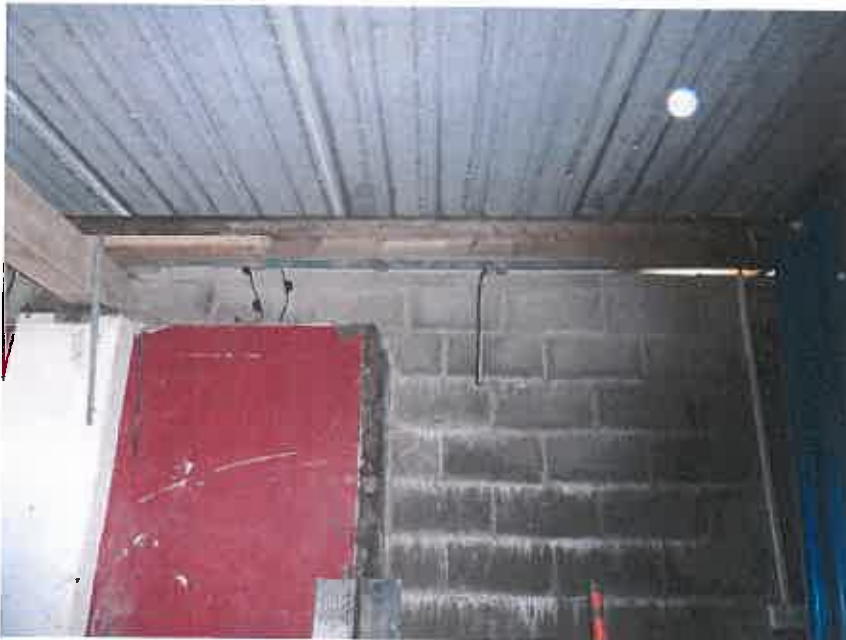
Photograph 5: Typical view of wide gaps behind fascia (east elevation) that lead directly into the building.
