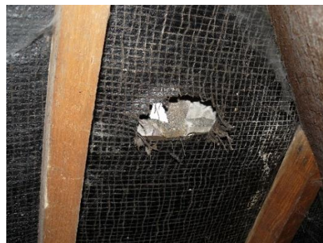
Figure 10: Hole in roof lining
