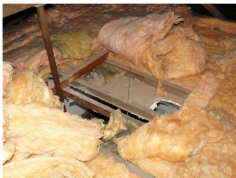
Figure 9: Hole in floor of loft space
