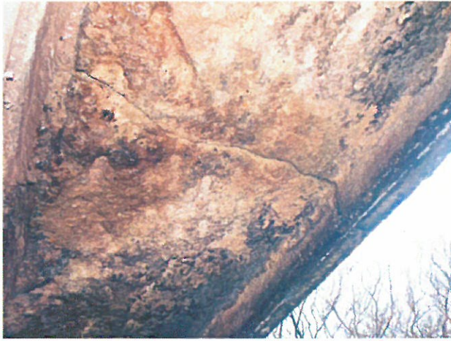
Image 009 (Visible crack on underside of lintel)
