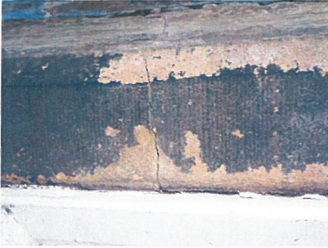
(Image 007, Cracking through stone lintel)
