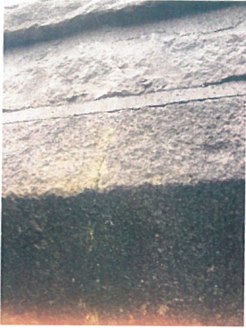
Image 011 (Crack visible from front face of lintel)
