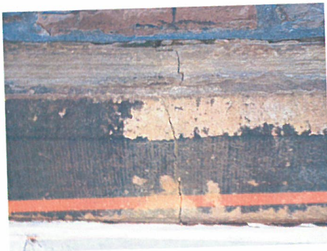
(Image 006, Vertical Crack running through
