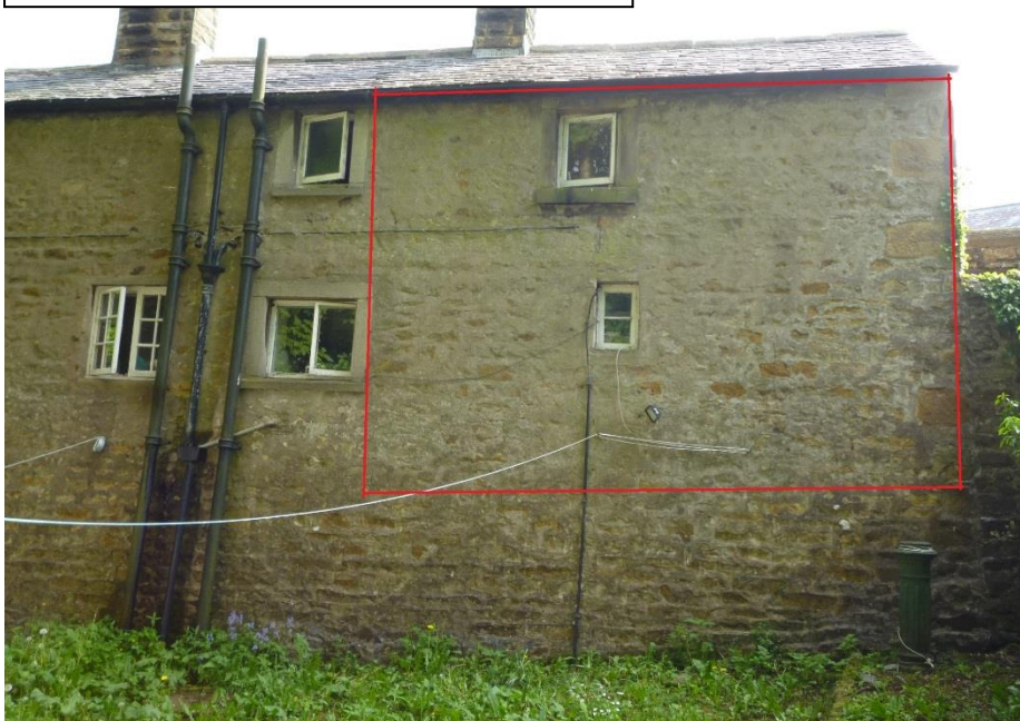
Photo 03 - Showing the slobbered render to the rear elevation inside the red highlighted area.
