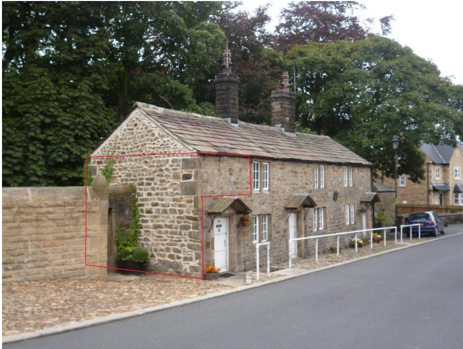
Photo 02 - Showing the front and side elevation to be repointed inside the red highlighted area.
