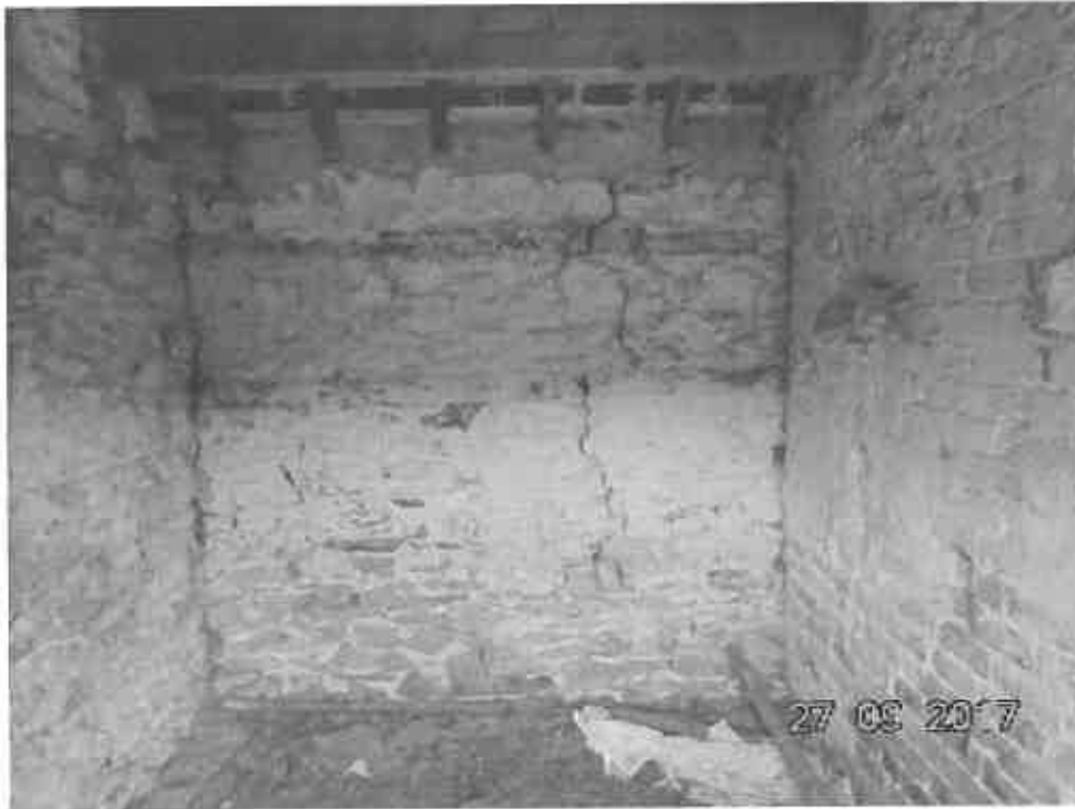
INTERNAL PIGGERY LEFT HAND SIDE
