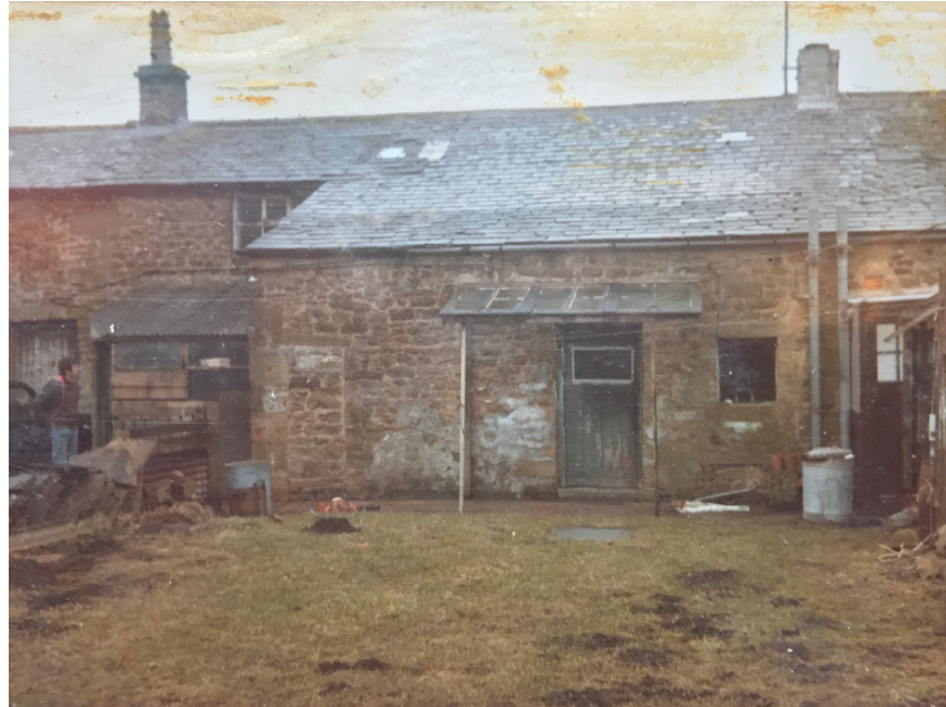
Figure 5 Rear view of the farmhouse in 1979 showing infill to the west and the annex before it was rebuilt
