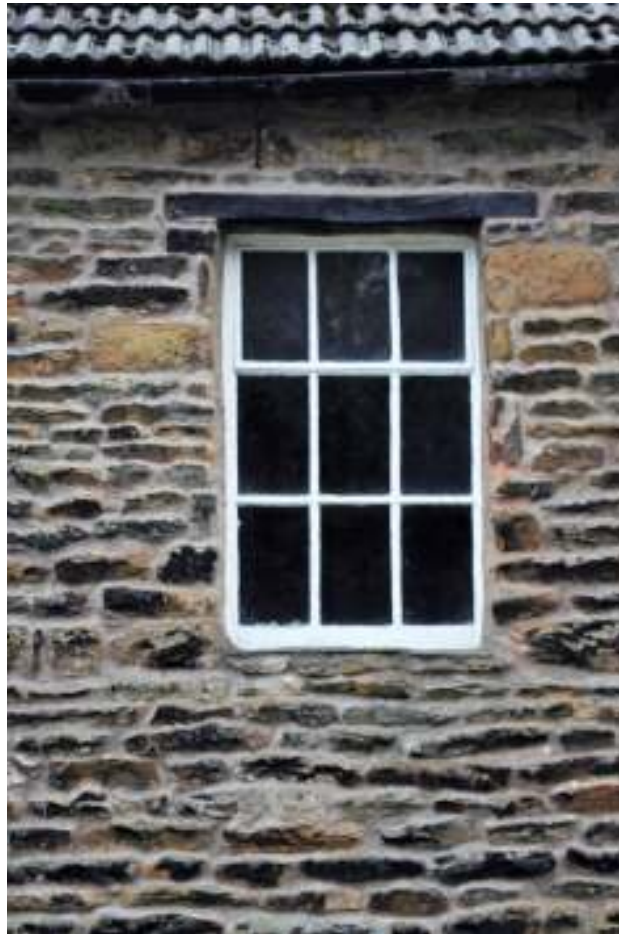
Figure 14. North elevation, FF2, second from right upper floor window.
