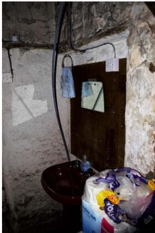
Figure 24. Blocked door to NW room of house, part hidden by panel and basin.
