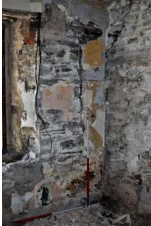
Figure 43. Masonry joint indicating blocking, south elevation window.
