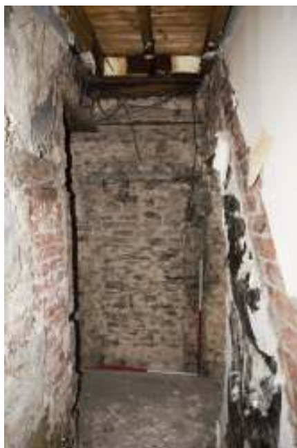
Figure 81. North west room, blocked door between south range rooms in east wall of passage through the staircase space.
