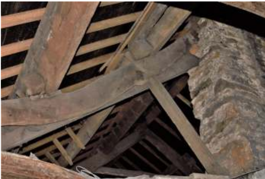
Figure 135 Packing pieces and support struts for modern rafters visible behind truss timbers.
