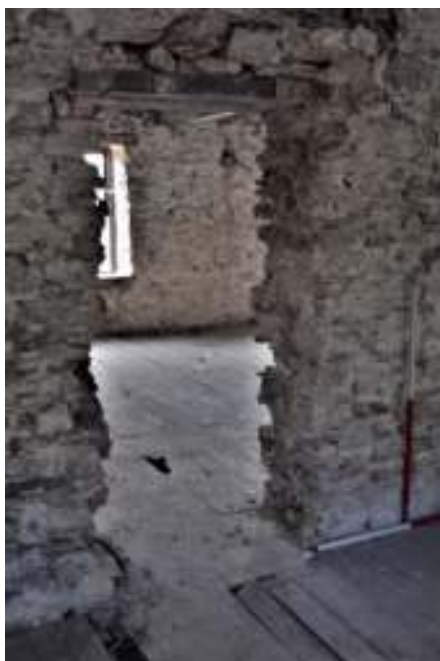
Figure 120 Doorway cut through spine wall to enable access between rooms partitioned from original spaces. For the use of PWA Planning and Mrs and Mrs McHugh.
