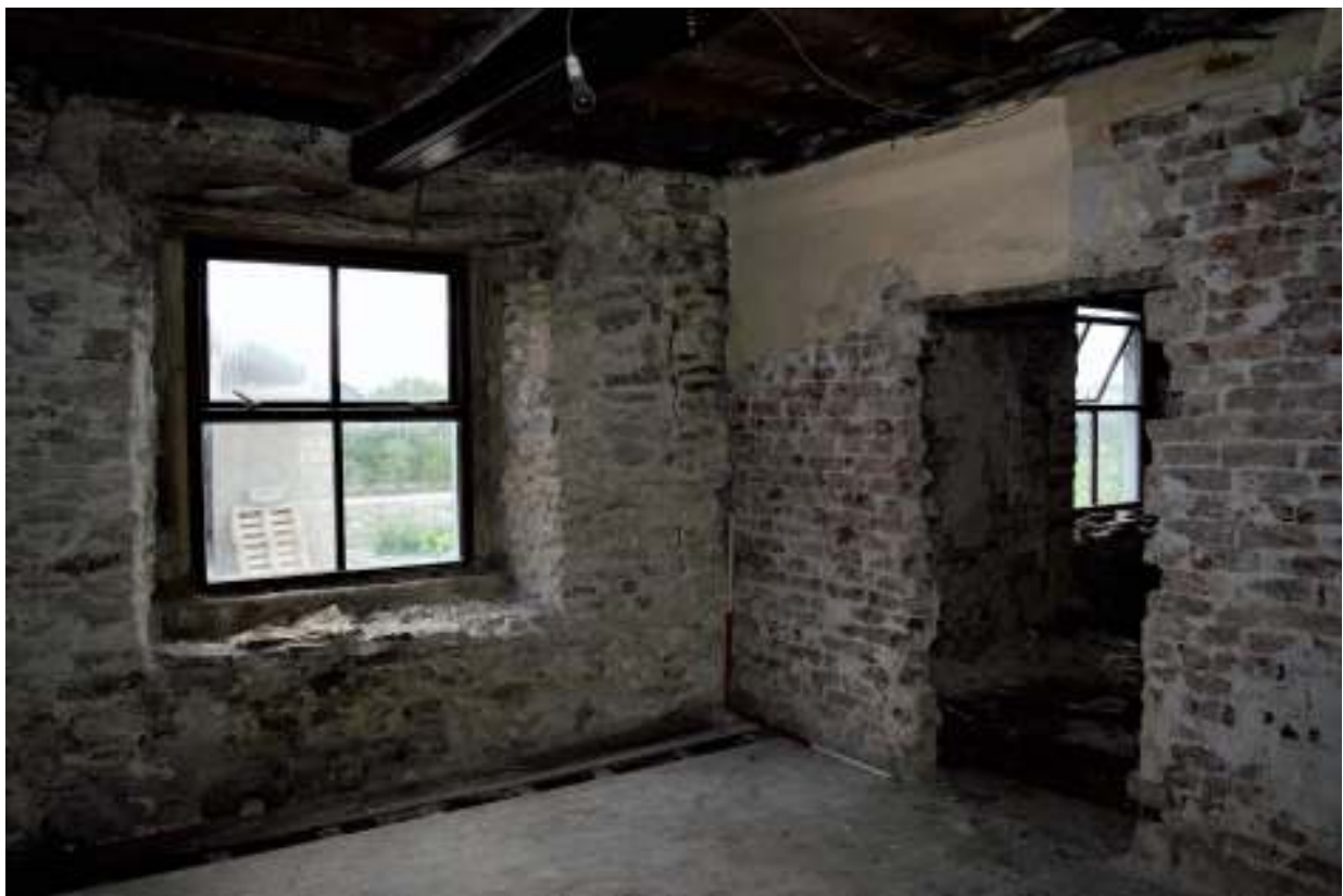
Figure 32. South east room door, south west corner with south window and inserted door in west wall.
