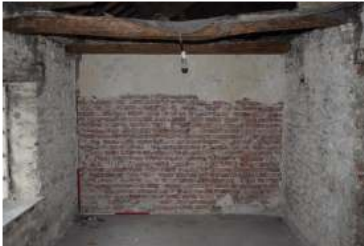
Figure 127. Upper north west room, inserted single skin brick east wall.
