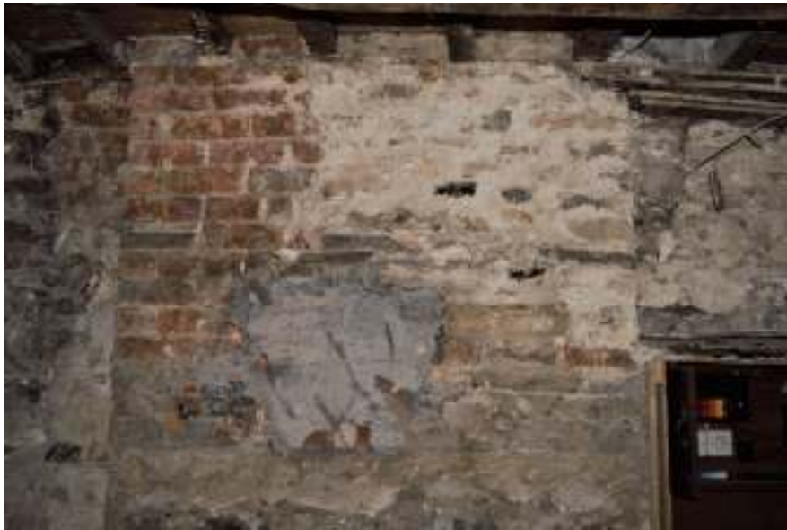
Figure 84. Blocked former sweeping hole in chimney breast.
