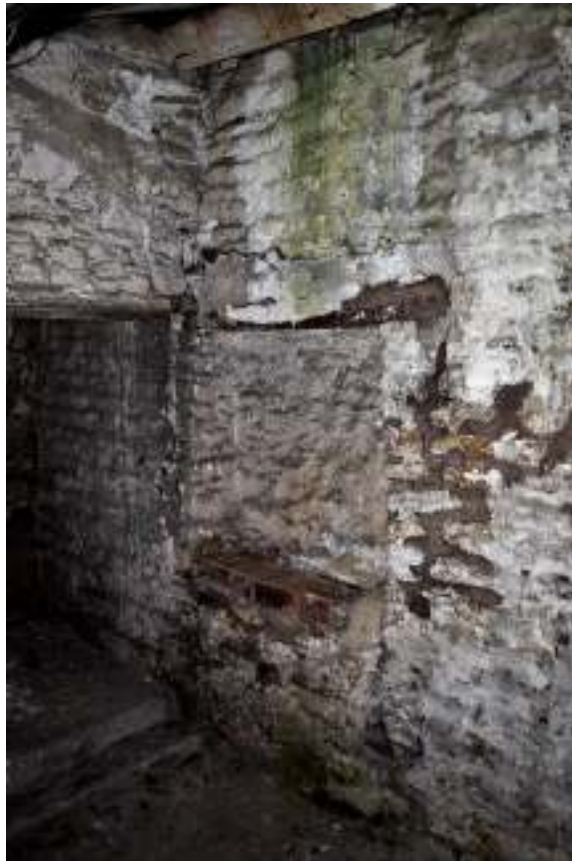
Figure 25. Blocked door to SW room of house.
