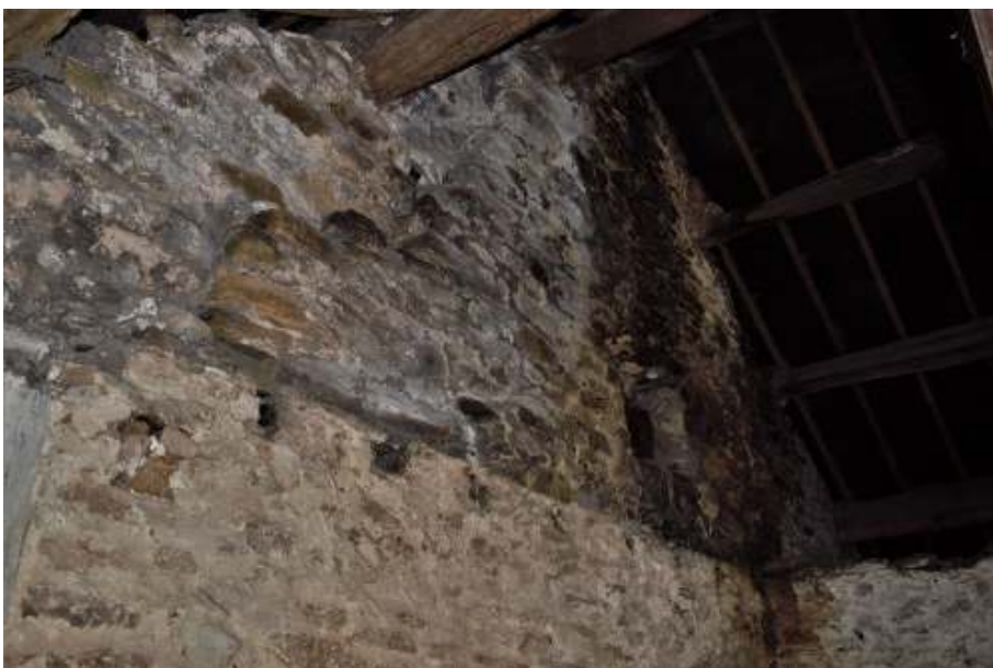
Figure 136 West gable wall with possible sweeping hole.
