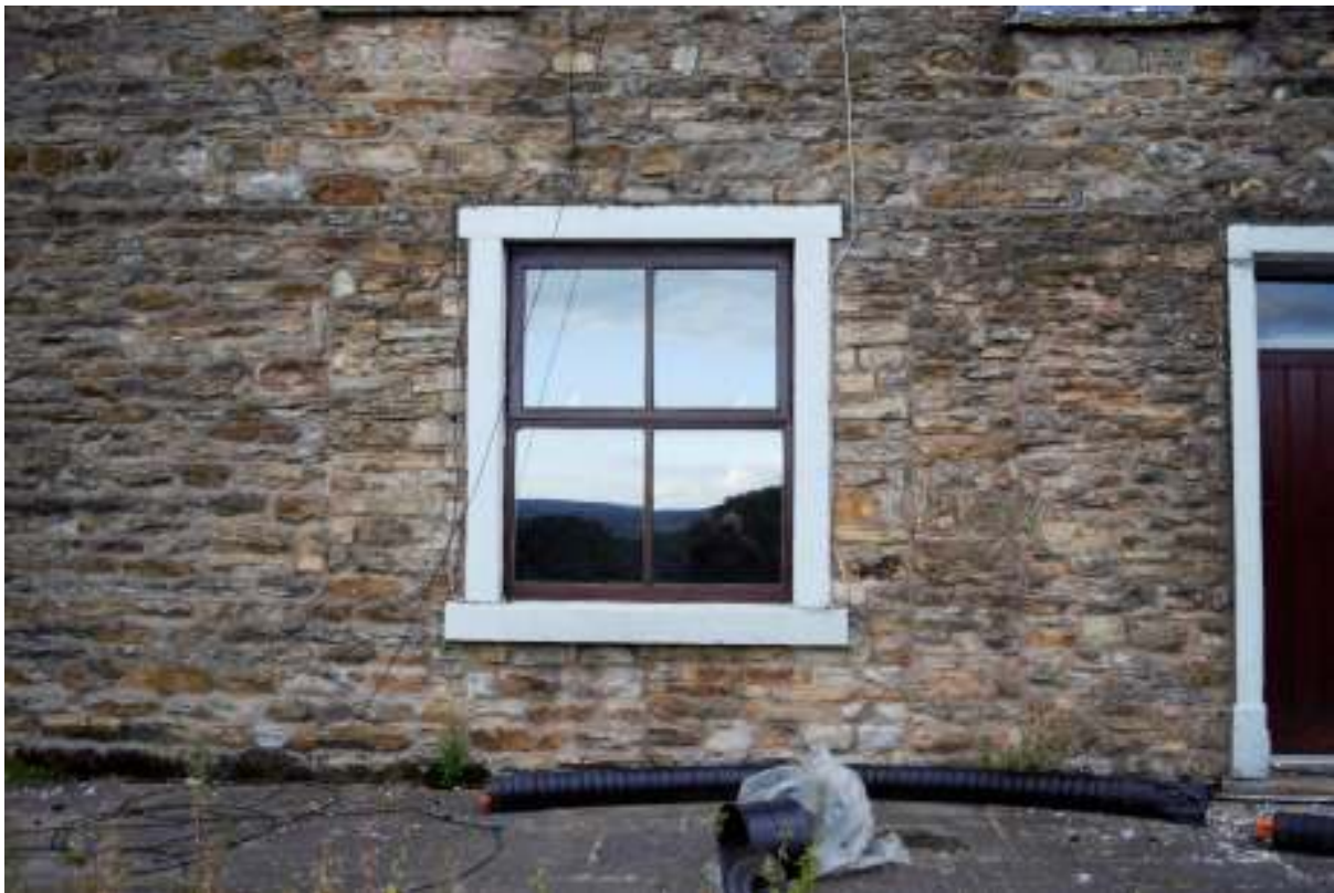
Figure 6. South elevation, ground floor window in reduced opening with blocked door to left.
