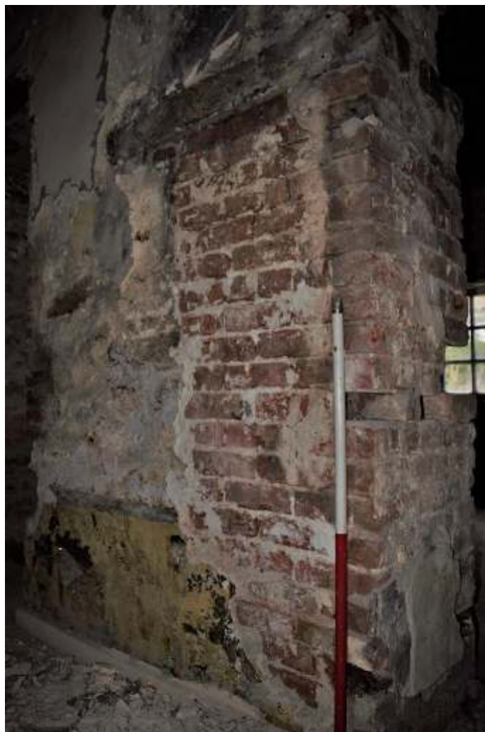
Figure 79. Northwest room, former stairwell, part blocking of original doorway and new opening to the east. For the use of PWA Planning and Mrs and Mrs McHugh. © MACCS January 2018
