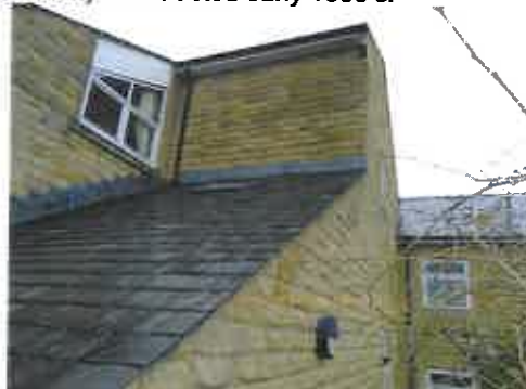
section of roof affected by construction of the lift
