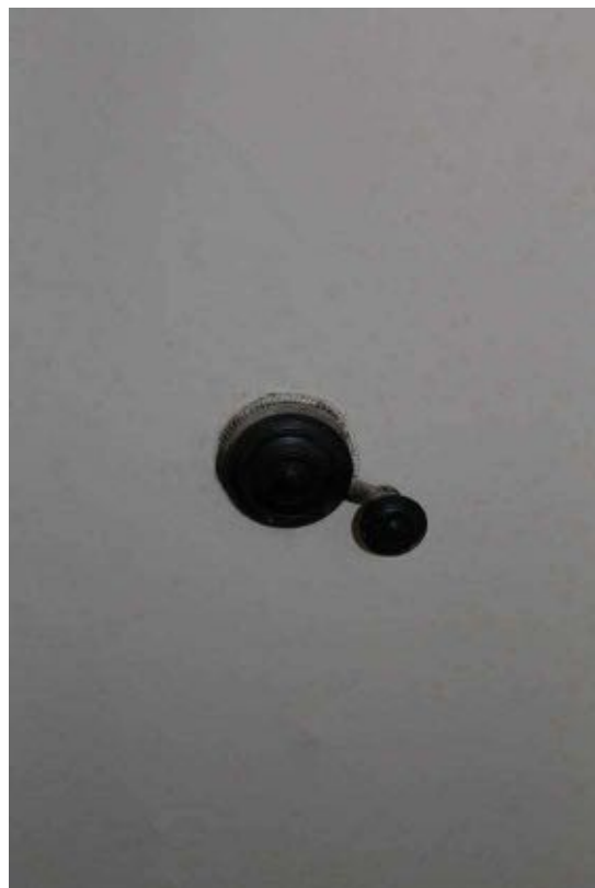
Plate 44: Service bell in corridor Room F18
