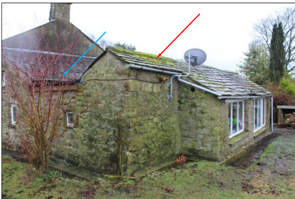
25. Rear of garden room, looking southwest, showing how it incorporates a small originally free-standing building, perhaps a privy (indicated by red arrow). To its left is the rear wall of the flat-roofed 1970s link (blue arrow)
