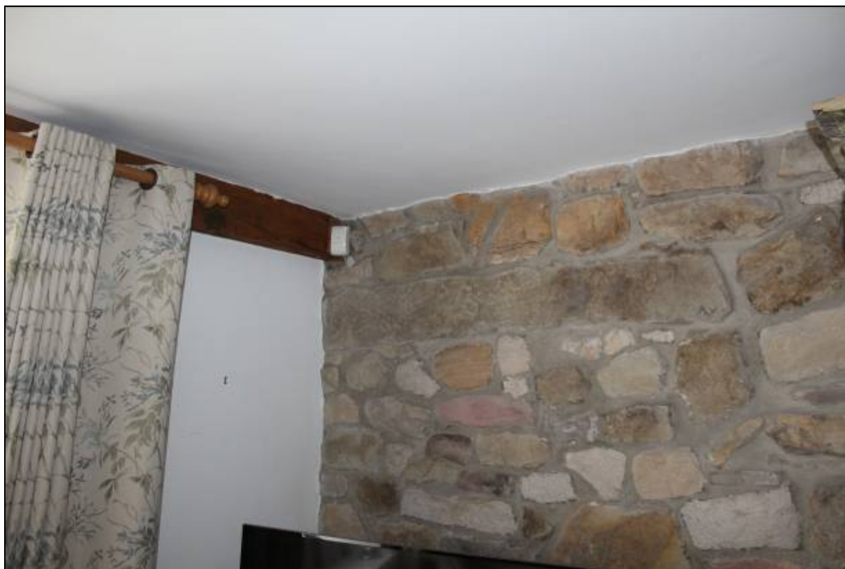
18. Evidence of blocked doorway to housebody in third bay of ground floor
