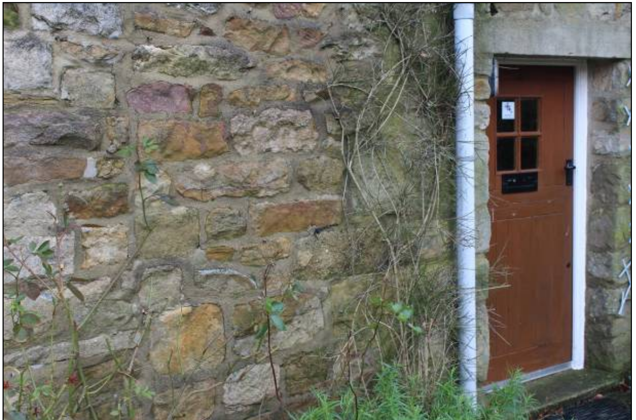
12. Evidence of blocked window at east end of main range
