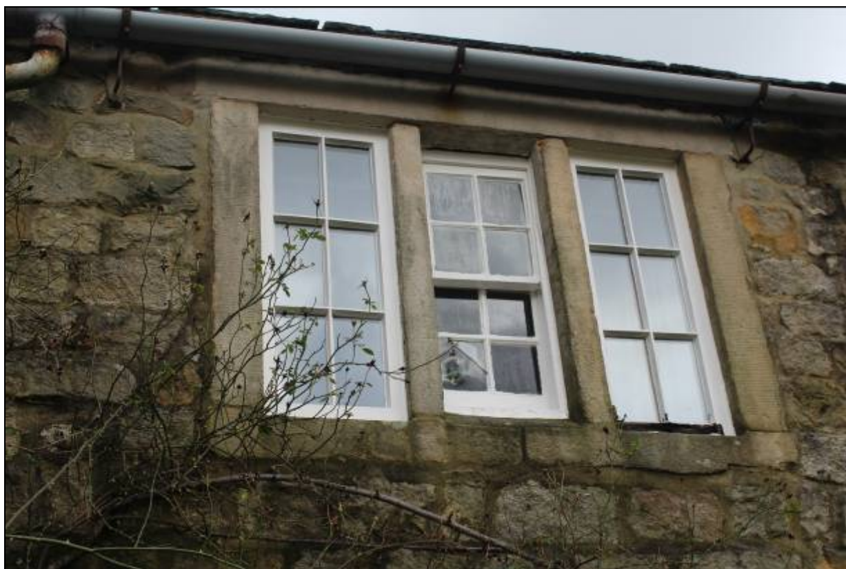
11. First floor window, showing 19 th century centre light glazing and late 20 th century replacements in outer lights
