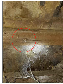
LH-1 View-2b Close-up of stone flag roof and nail fixing through batten
