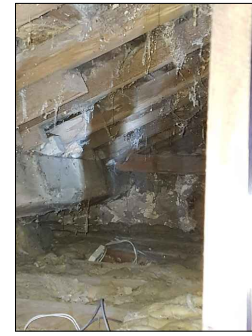
LH-1 View-4 Stone (west) gable wall and chimney (Bed-3) at loft level.
