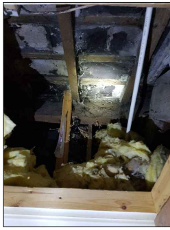
LH-1 View-1 Slate roof finish nailed to fixed battens (north facing/ rear elevation),
