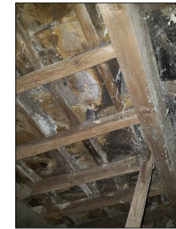
LH-2 View-4 Stone flag roof finish nailed fixed to battens, no felt/ membrane (south facing/ front elevation),
