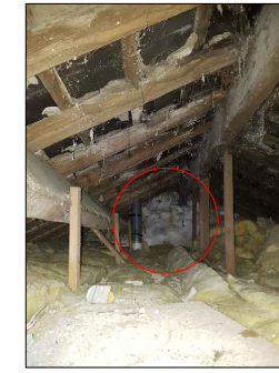
LH-2 View-1 Lime render plastered east gable wall (bathroom) at loft level.
