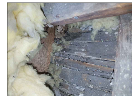
LH-2 Ceiling Lath and plaster ceiling from loft level (over Bed-1, Bathroom & Wc) - refer to other images for apparent plasterboard underdraw
