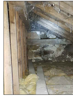
LH-1 View-3 Stone (west) gable wall and chimney (Bed-3) at loft level.
