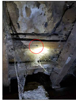
LH-1 View-2a Stone flag roof finish nailed to fixed battens (south facing/ front elevation),
