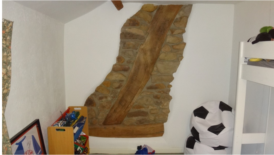
Figure 1 Part cruck frame in west wall of central bay towards the front of house at first floor
