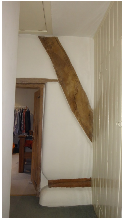
Figure 2 Part cruck frame in west wall towards rear wall of central bay of house on first floor landing; partly concealed by a later airing cupboard and; broken by the insertion of a doorway
