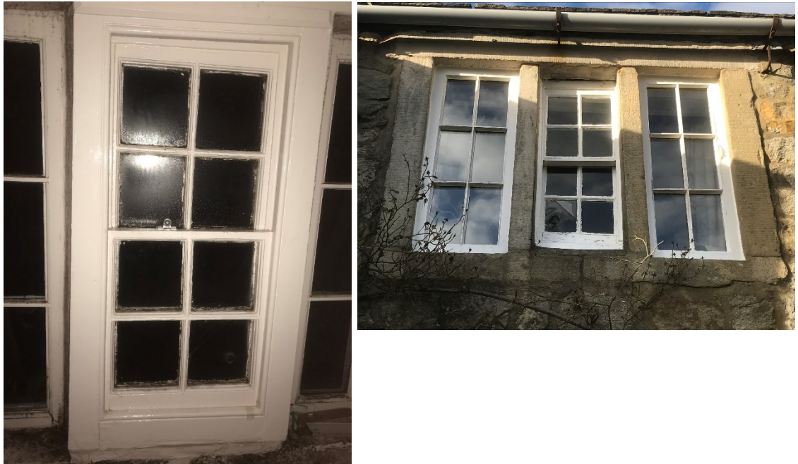
Figure 7 Existing sliding sash in the centre of the 2 squared mullioned window WF01 to be retained – paint stripped, and cords and sashes put back to working order. Cement pointing replaced with compatible mastic
