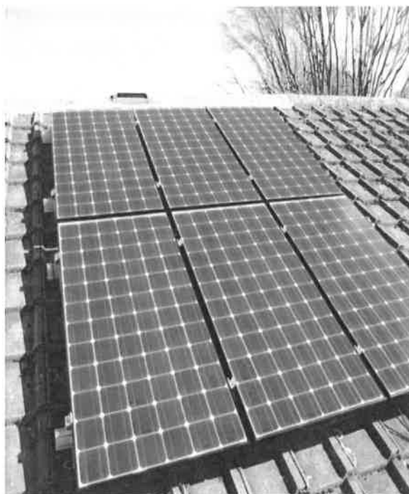
Figure 7 - Photovoltaic array on a pitched roof
