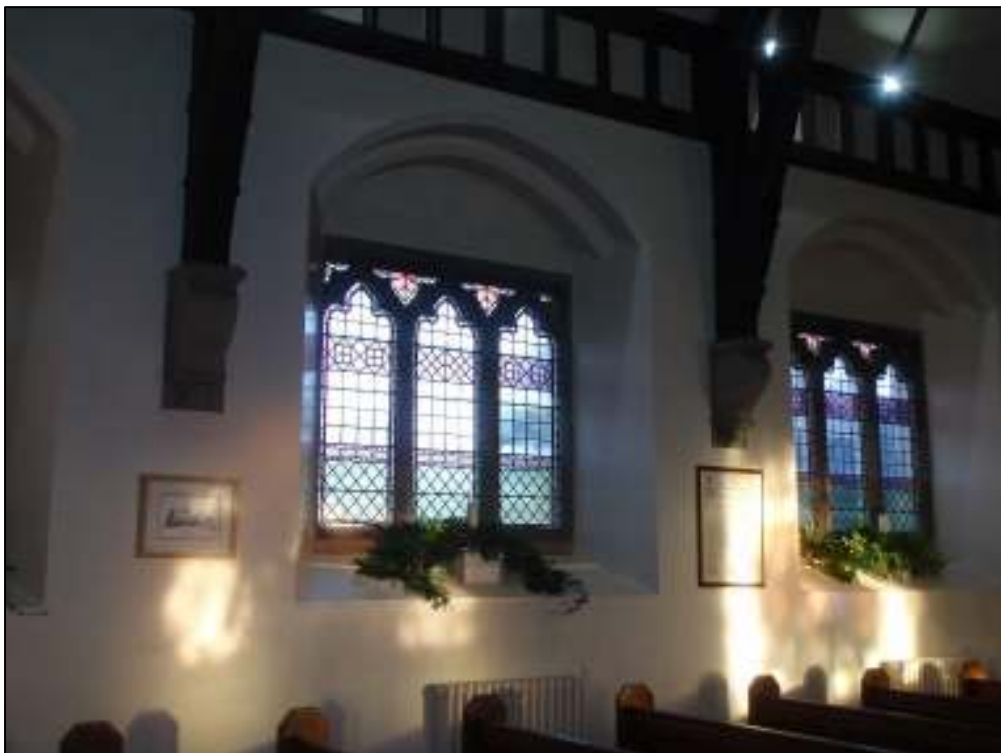
23: The second window in the north wall, counting from the west. This window will be removed to enable access from the main church building to the proposed development. The panes and their surroundings were well fitting, with no opportunity for bat access noted
