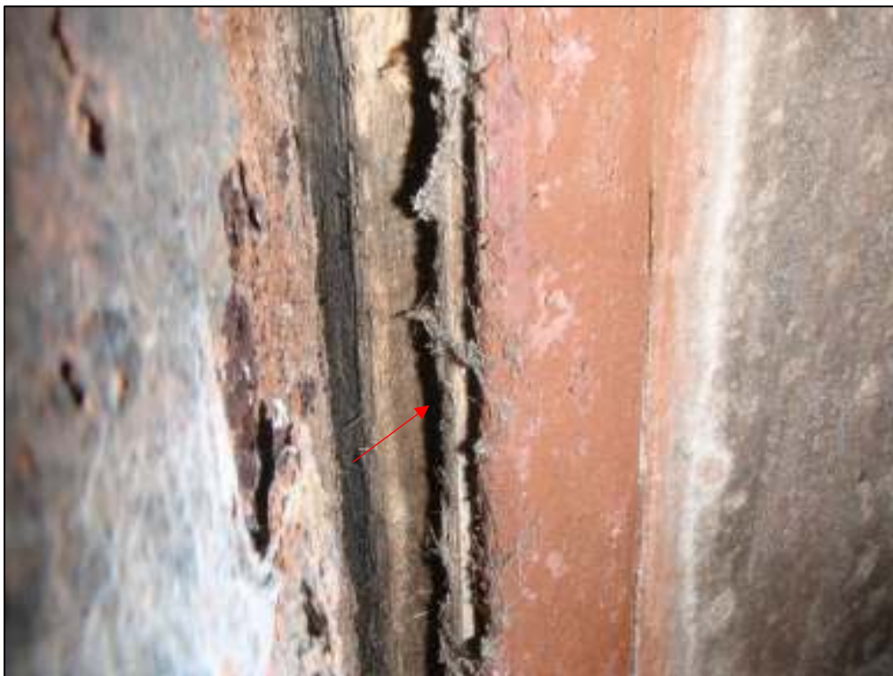
12c: Gap between soffit boards on right and guttering on left, marked by arrow, potentially leading into roof space
