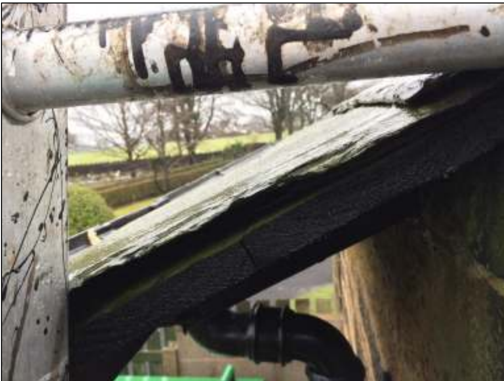
11: Sizeable gap under roof tiles at west end of the kitchen, creating potential roost space
