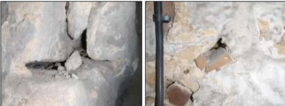
18a and 18b: Examples of cavities in the east wall of the boiler room, giving access into the wall space
