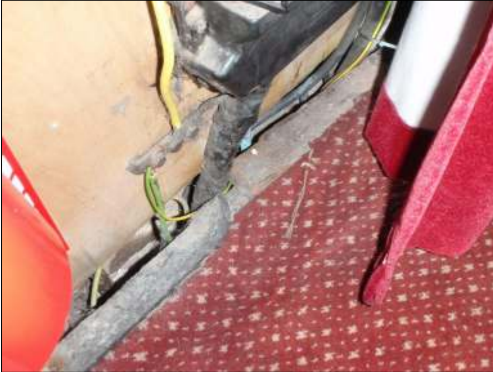
26: Access point into the undercroft where electric cables pass through floor, by the Churchwardens' pew in the south-west corner of the main church building
