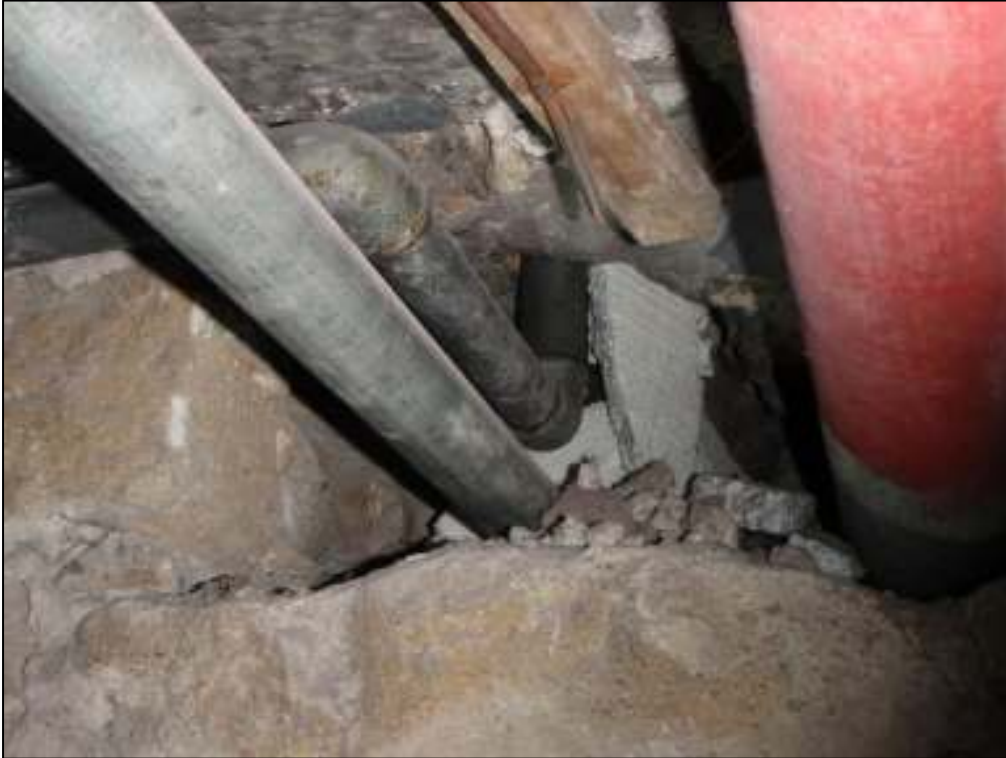
17: Pipework entering the west wall of the boiler room. Insulation in the pipework cavities consisted of pieces of polystyrene rather than expanding foam type insulation, allowing potential bat access into the walls
