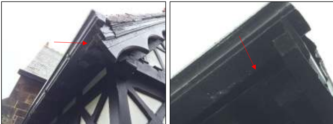
14a and 14b: Example of a large gap behind soffit, providing a potential access point into the roof space, at the south-west corner of porch on south side of main church building
