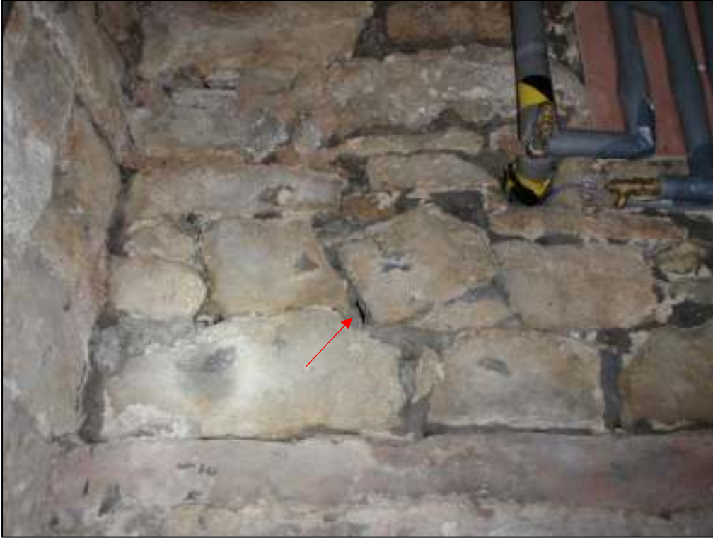
19: Wall in the side cellar, with cavities between stones providing potential bat access into the wall
