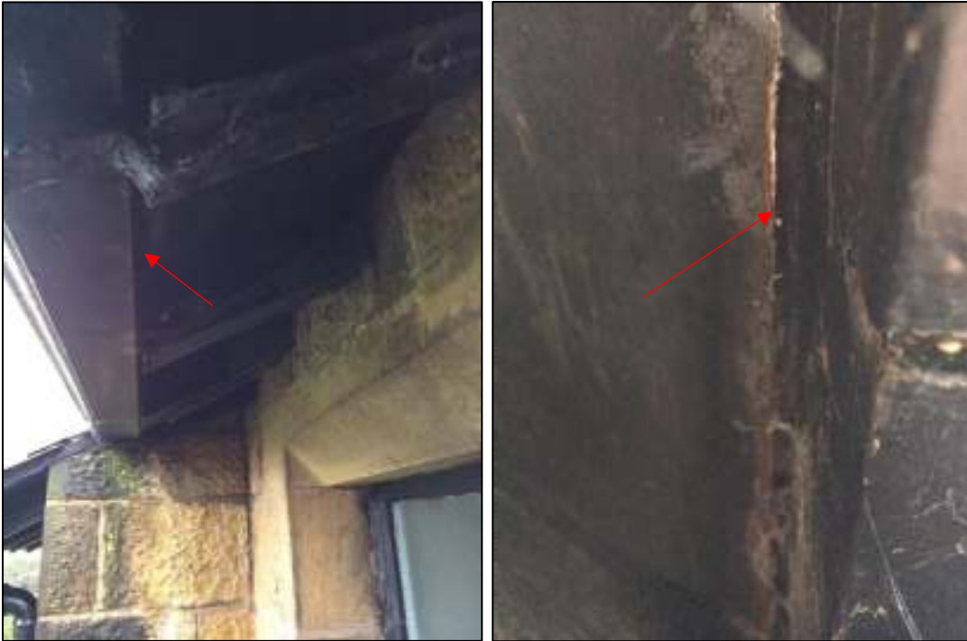
10a and 10b: Probable gap behind soffit along north side of kitchen roof, where soffit abuts guttering rather than fascia boards. 10a taken looking east, 10b taken looking west
