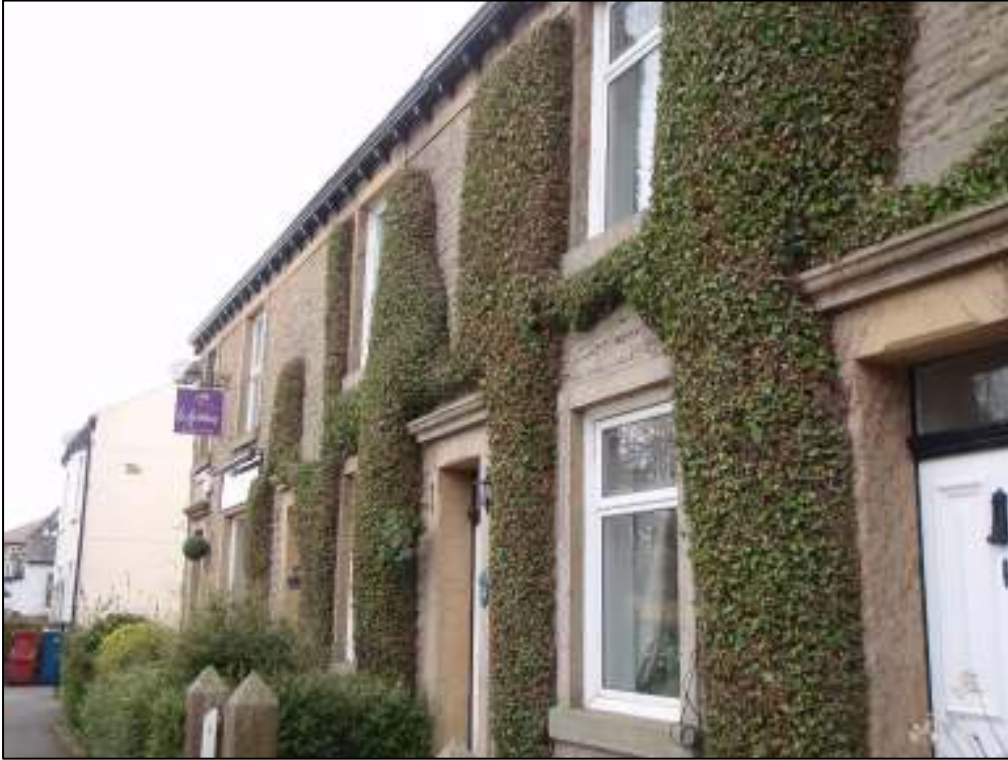
31: Part of the row of terraced houses on the west side of Lovely Hall Lane, opposite the church. No checks for PRFs were carried out here, but it was noted that the dense shrubbery on the walls offered shelter and potential roosting habitat for bats
