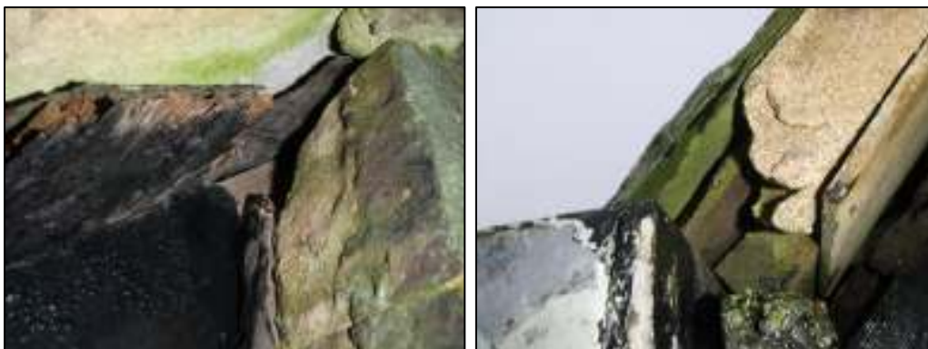
1b and 1c: Close up view of the two gaps above bargeboards at the north-west corner of the western gable end
