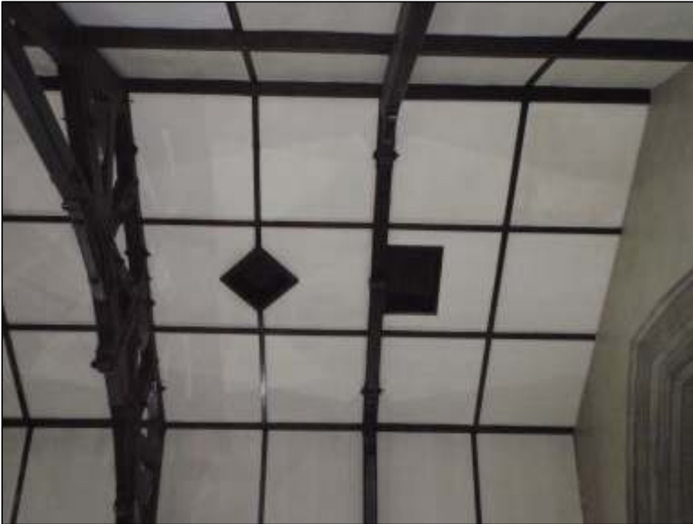
24: Two hatches leading into the upper roof space and providing access to the church spire. These were not accessed during the bat roost suitability survey, as scaffolding would be required
