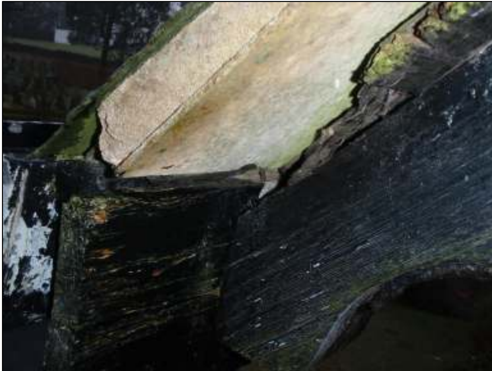
1a: Two gaps above bargeboards at the north-west corner of the western gable end
