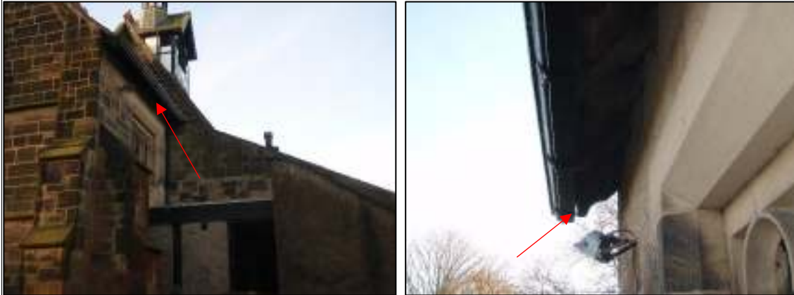
12a and 12b: Main church roof at north-east corner of church, with loose-fitting soffit creating gap between guttering and soffit boards. The gap can be seen against the sky in photograph 12b (marked by arrow)
