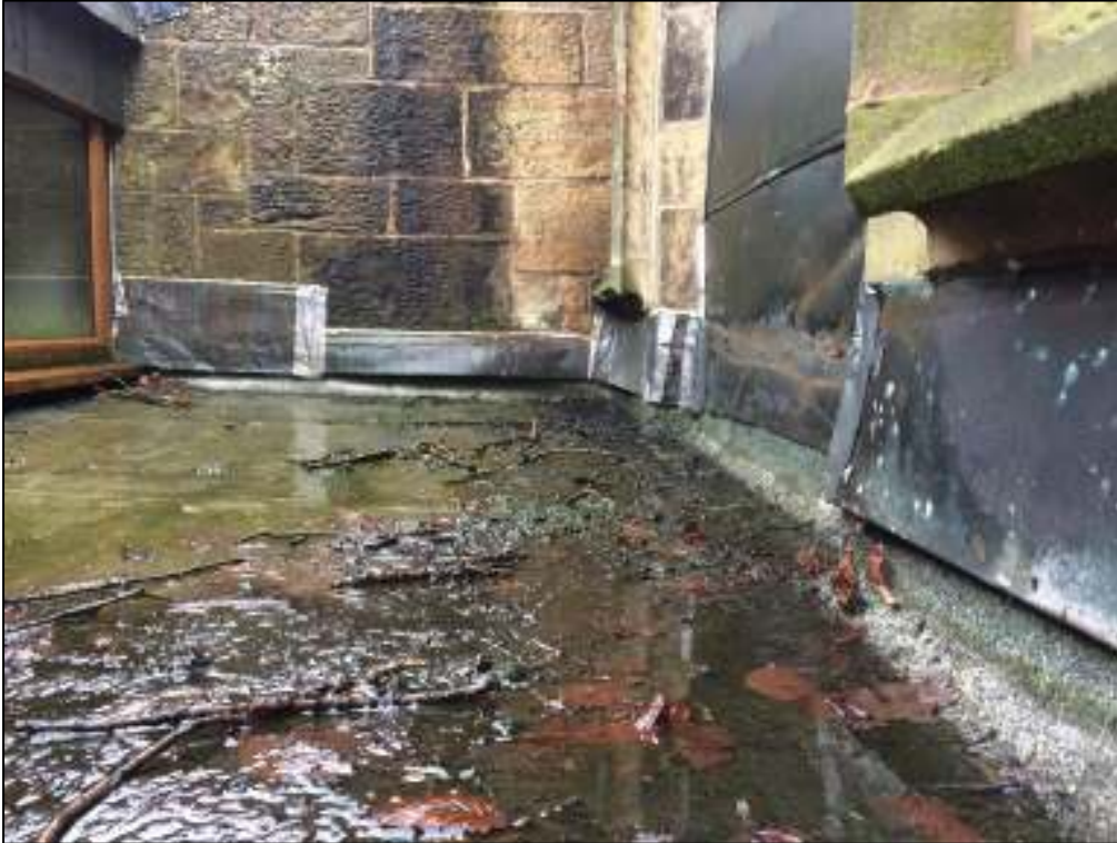
5: Lead flashing lifting in several places above the small flat roof between the choir vestry and the main church building
