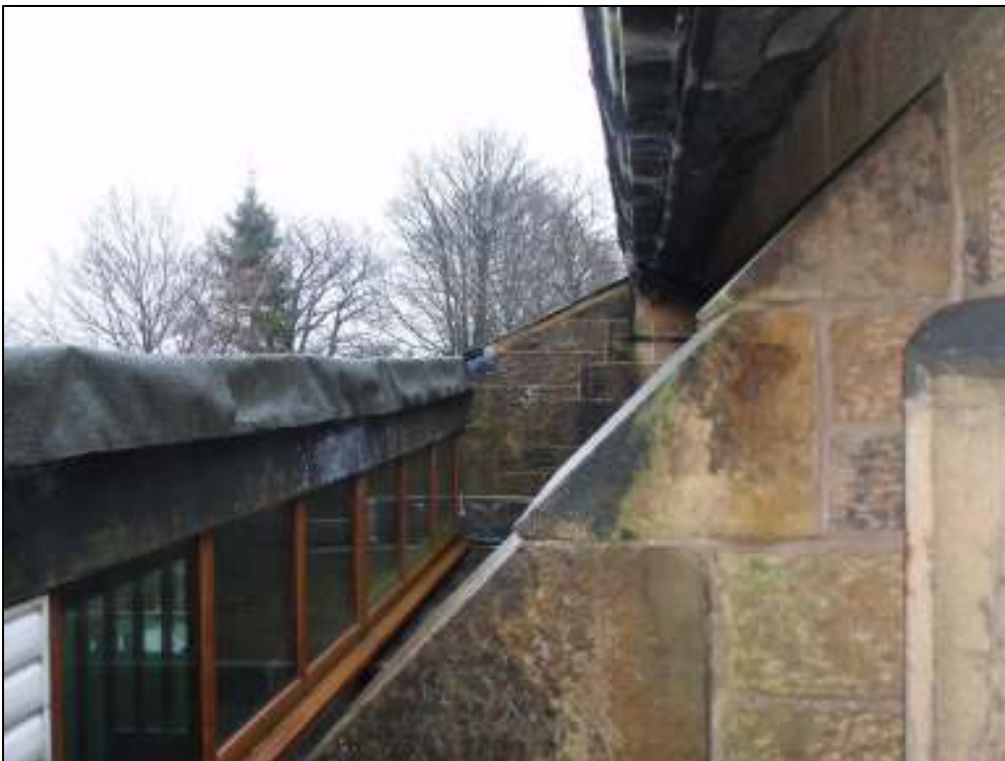
3b: looking along the gap between the main church roof (on the right) and the choir vestry roof (on the left). PRF 3 is located under the guttering/soffit of the main roof on the right; PRF 4 is located under the roof felt on the choir vestry roof on the left
