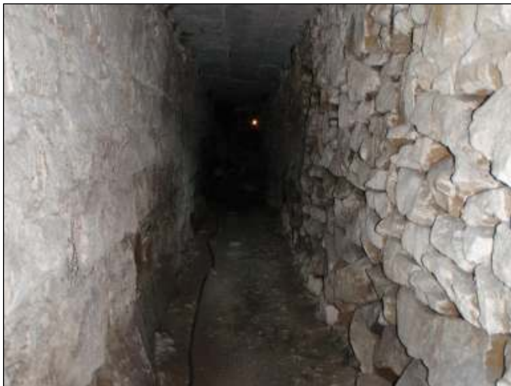
21: Looking along a section of the undercroft. The wall on the right, without extensive pointing, was typical of some areas and provided PRFs for bats and, in places, cavities accessing the wall spaces
