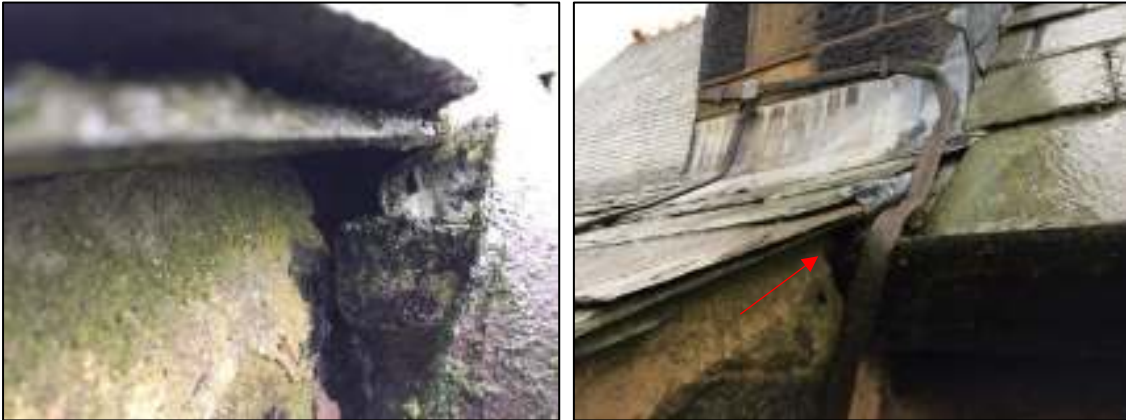
6c and 6d: Access point into roof underneath tiles, at join between main church building and kitchen area, above the south-east corner of the flat roof behind the choir vestry
