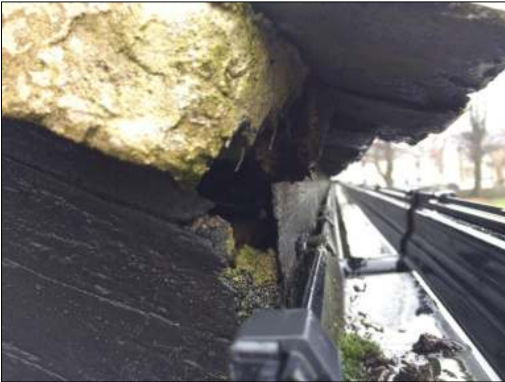
8: Hole in rotten fascia board at north-east corner of choir vestry roof, accessing cavity under roof tiles running along the north side of the choir vestry
