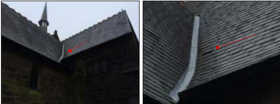
13a and 13b: Example of lifting roof slate on the main church roof, to the east of the Lady Chapel
