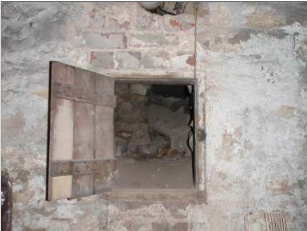
20: Door leading from the side cellar into the undercroft. This door was ajar at the time of the survey, and other cavities around the pipework etc. suggest that bats could move between the undercroft and the cellars
