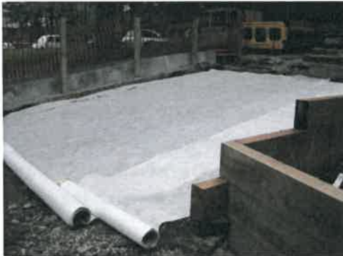
Laying of geotextile fabric with the cellular confinement system pinned in place
