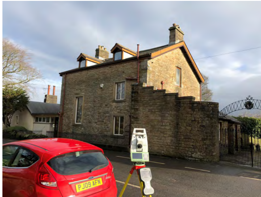
Road side elevation including parapet wall to lean to extension - made because of water ingress, entrance to courtyard
