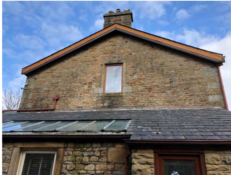
Existing lean-to extension roof, rooflights and blocked up window to side elevation.
