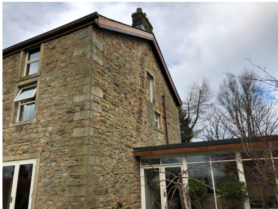
View from garden showing connection of hallway and original house as well as blocked up window to side elevation
