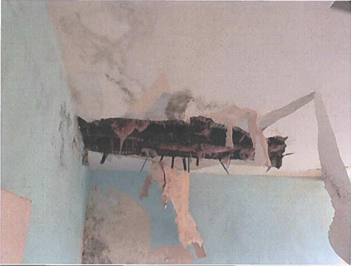
Example of damage to first floor ceilings
