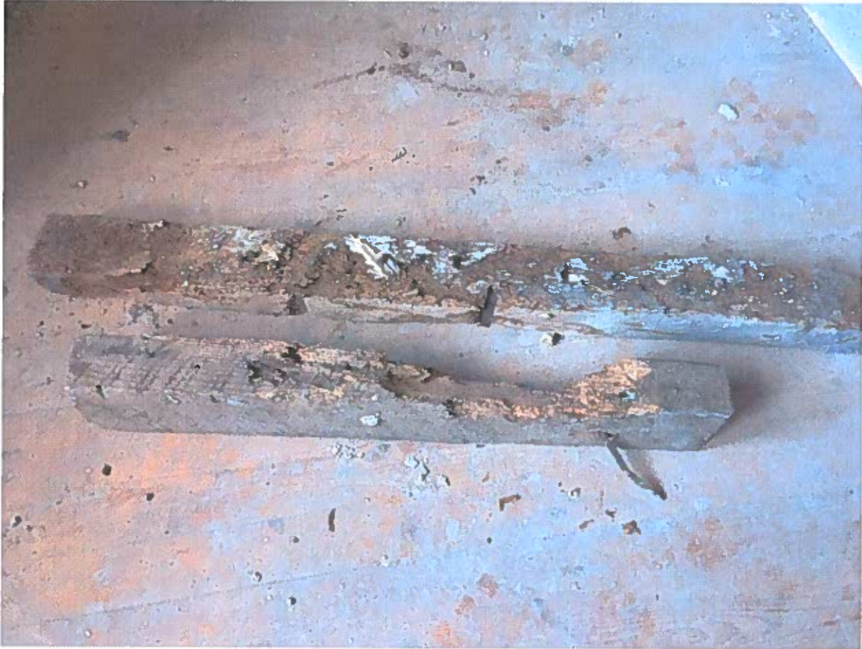
Example of rotted and woodworm damaged roof timbers
