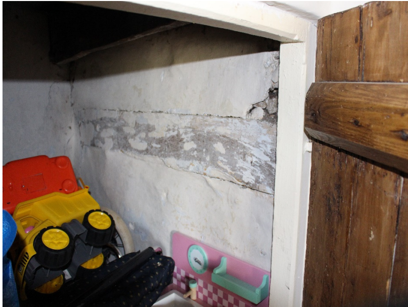
Photograph N0.2 showing timber in wall below the stair landing.
