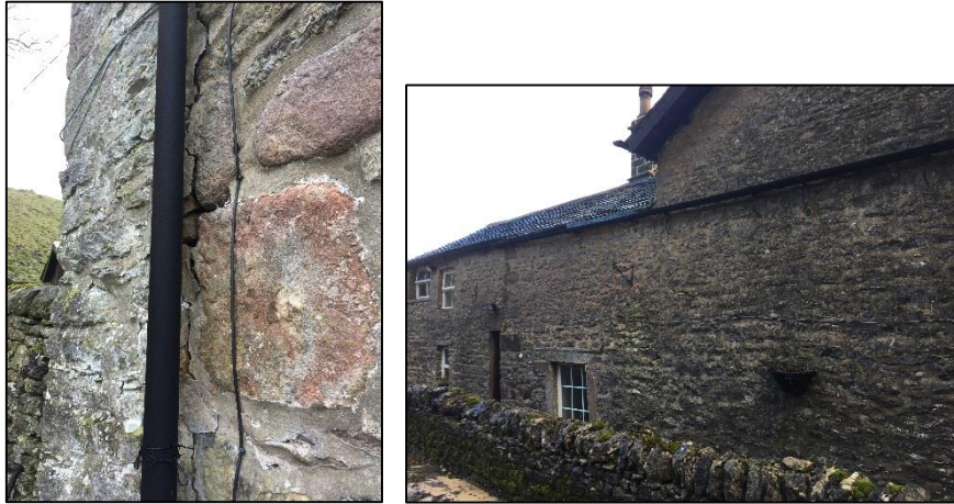
Plates 7 & 8: Gap in mortar on eastern elevation and southern elevation to be re-built
