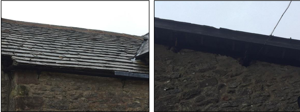
Plates 3 and 4: Missing & raised roof tiles & gaps in masonry at eaves of building.
