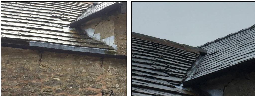
Plates 5 and 6: Structural crack and gap beneath ridge tile at top of valley gutter
