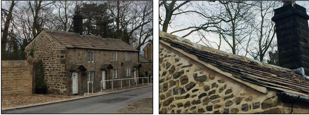
Plates 1 and 2: North-west and eastern elevations of farmhouse & lifted lead flashing
