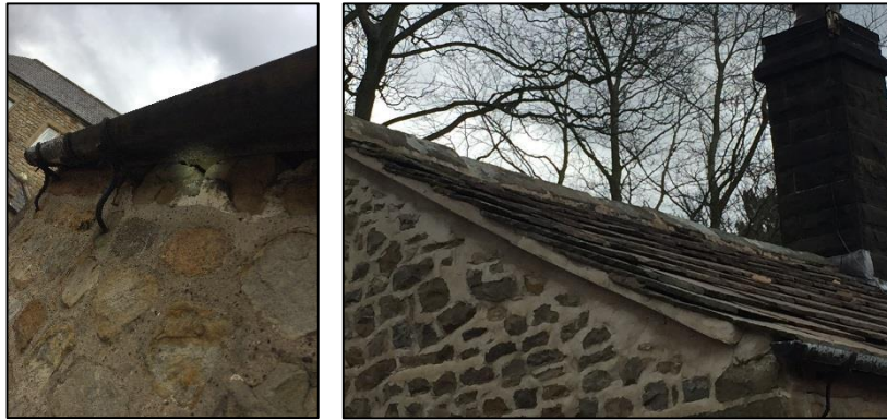
Plates 3 and 4: Gaps on wall tops & gaps beneath tiles on northern gable end
