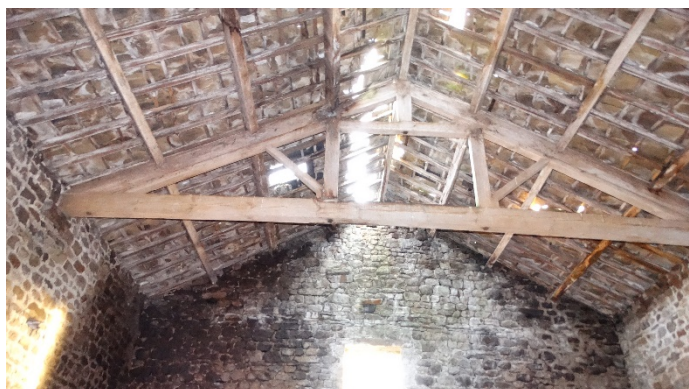
Figure 3: SE gable end of barn showing roof damage
