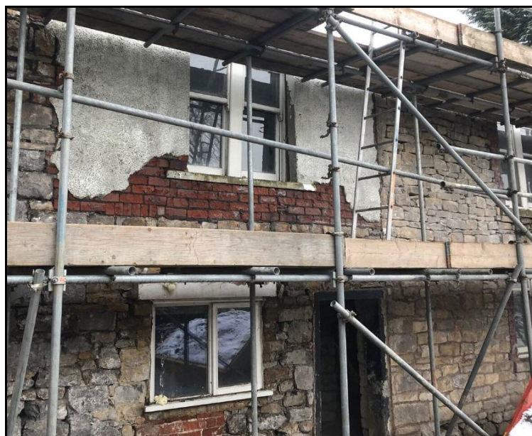
Figure 8) Rear elevation during render removal showing full height joint right of doorway and partial brick walling at first floor and beneath the ground floor window.
