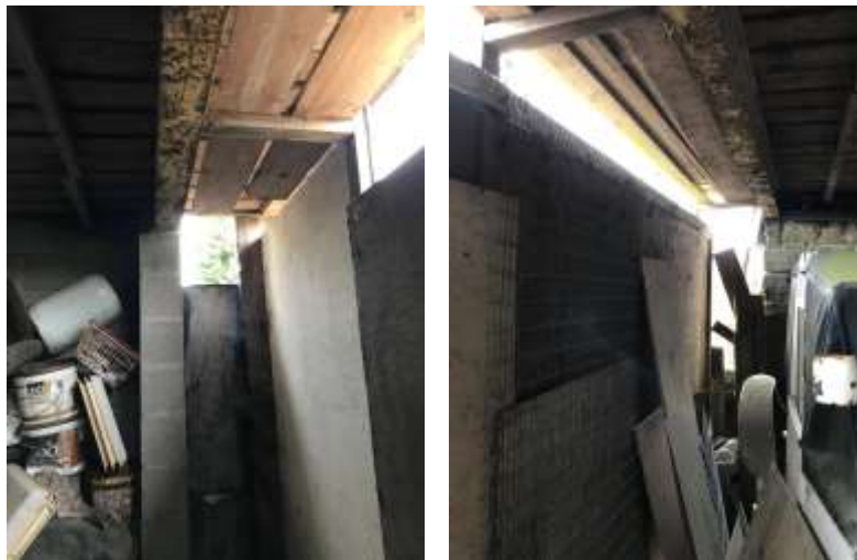
PL. 8. Illustrating section of ad-hoc timber framed infill providing some protection to where the front North facing section of the agricultural outbuilding wall has been removed previously.
