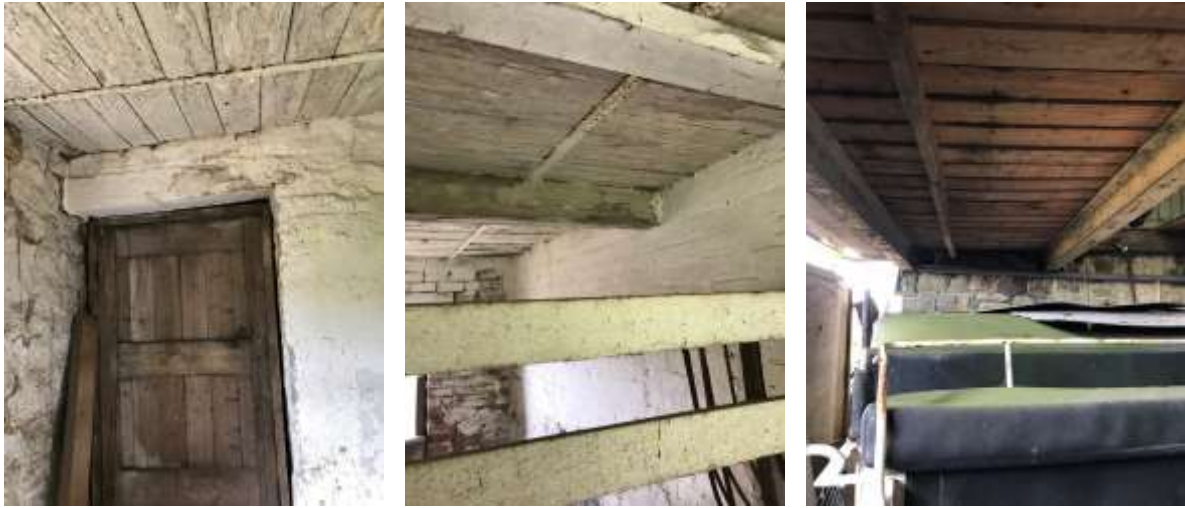
PL. 18. Timber boarded floor supported by timber joists and intermediate metal bracing straps within part of the main Barn.
