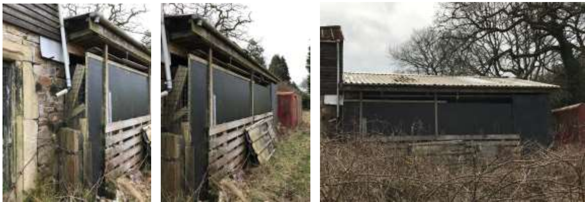
PL. 12. Illustrating section of ad-hoc timber framed infill providing some protection to where the front North facing section of the agricultural outbuilding wall has been removed previously.
