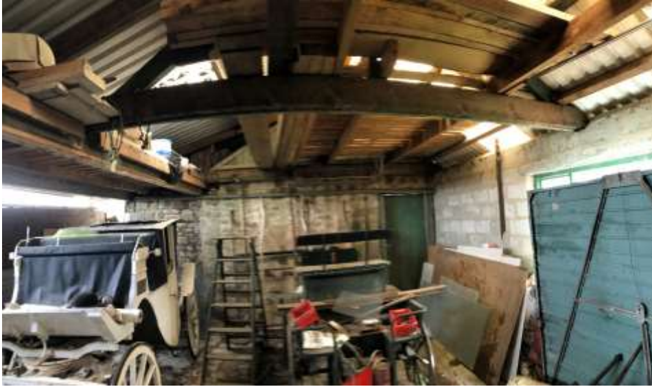
PL. 5. Illustrating existing roof structure (Trusses, timber purlins/sheeting rails) centrally over adjoining agricultural Outbuilding facing West.
