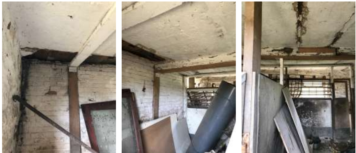
PL. 19. Cement/plaster finishes prevented part of the existing first floor structure over the main Barn from being clarified. Potentially suspended concrete but more likely to be again timber boarded floor supported by timber joists and intermediate metal bracing straps within part of the main Barn. Further intrusive investigations required.
