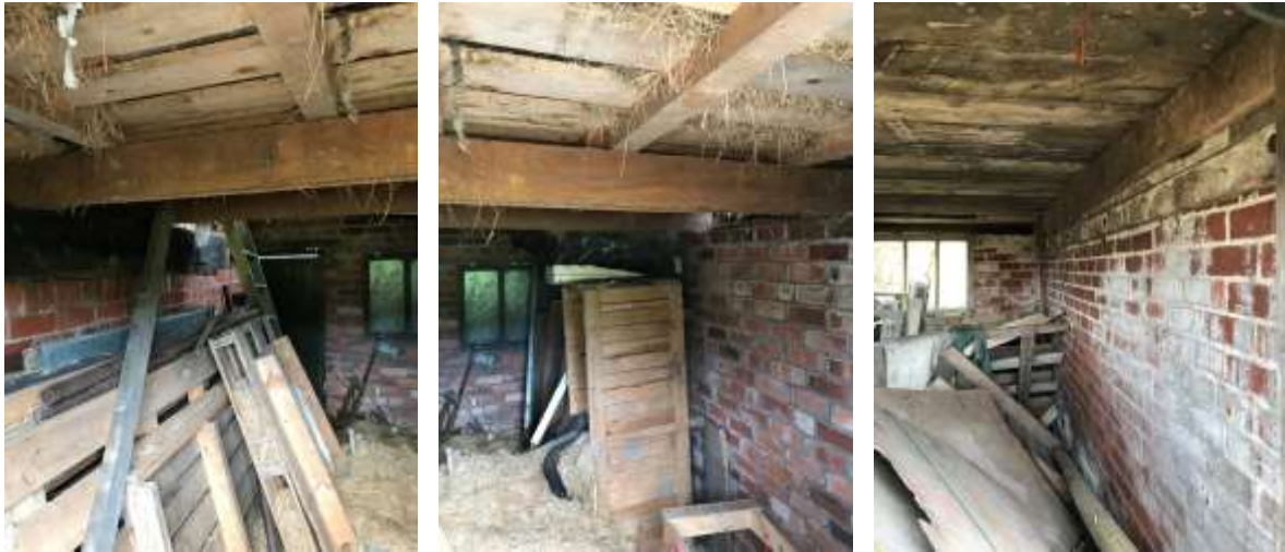
PL. 20. Timber boarded floor supported by timber joists and intermediate metal bracing straps within part of the main Barn.
