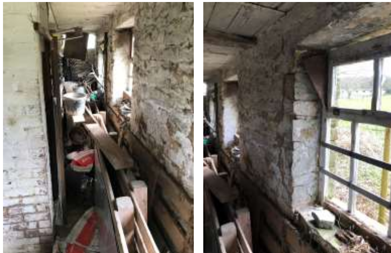
PL. 15. Illustrating internal faces of external masonry walls present at the time of inspection. Generally walls appeared sound, true and level with no significant bowing or undulations noted. Also walls appeared free from any significant and obvious structural movement. In addition, window and door heads generally appeared true and level.
