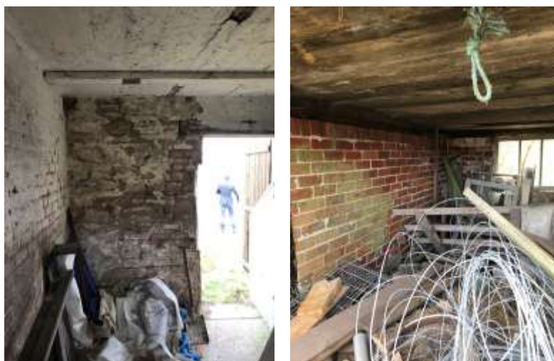
PL. 16. Illustrating internal masonry walls present at the time of inspection. Generally walls appeared sound, true and level with no significant bowing or undulations noted. Also walls appeared free from any significant and obvious structural movement. In addition, window and door heads generally appeared true and level.ss
