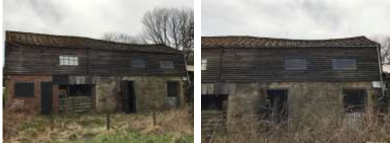
PL. 2. Illustrating corrugated cement asbestos sheet roofing covering to that of the North facing roof pitch of the main Barn.
