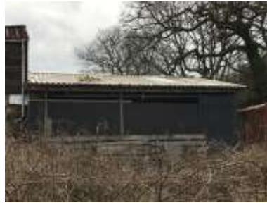
PL. 3. Illustrating light weight metal sheet roofing covering to that of the adjoining North facing agricultural Outbuilding structure.
