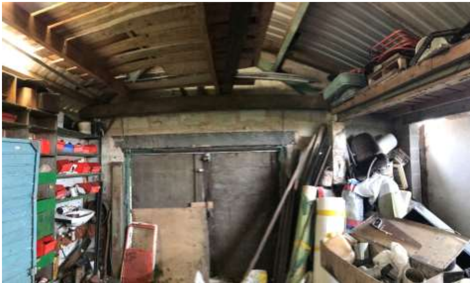
PL. 4. Illustrating existing roof structure (Trusses, timber purlins/sheeting rails) present within the adjoining agricultural Outbuilding facing West.
