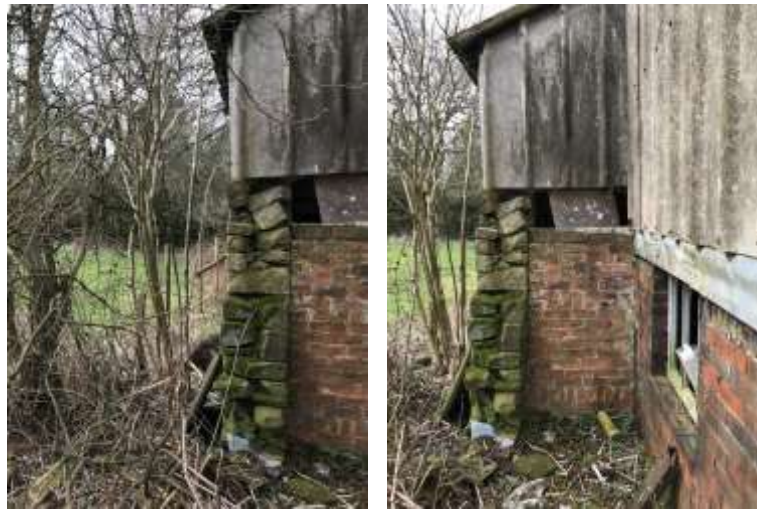
PL. 9. Illustrating section of stone work to be made good and re-built.
