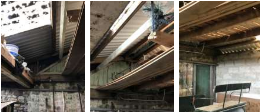
PL. 6. Illustrating existing roof structure (Trusses, timber purlins/sheeting rails) present within the adjoining agricultural Outbuilding facing East to party wall with that of the main Barn.
