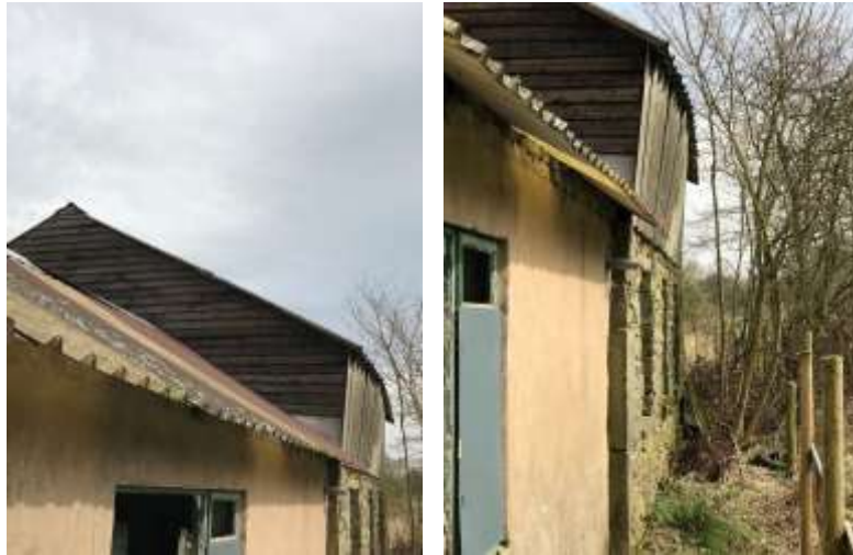
PL. 14. Illustrating the warped timber frame and cement asbestos sheet cladding present to the South facing elevation of the main Barn.
