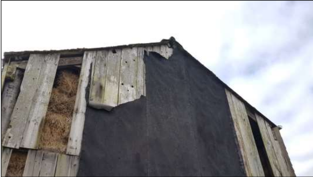
Plate 5: The gable east end of the main barn. Large holes exposed due to missing timber beams.
