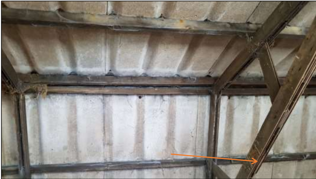
Plate 7: The structural beams of the barns had slotted gaps which were potential bat roost structure.
