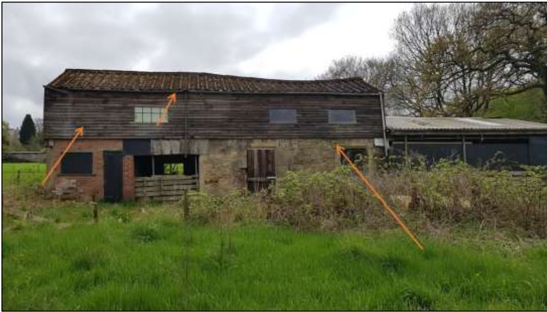
Plate 4: View of the barns from the northern side of the building. The arrows show gaps between stones on the barn and exposed gaps underneath tiles due to lack of fascia. The weatherboard is highlighted to show where gaps are.
