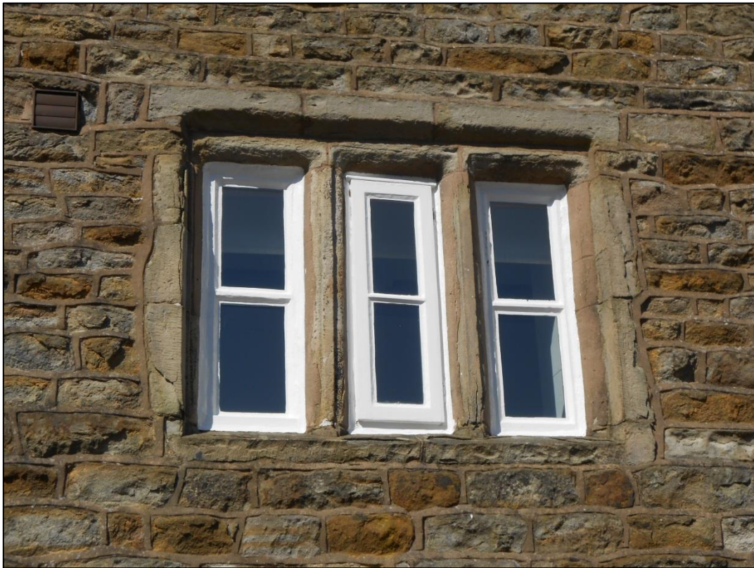
PL00: Window present to the first floor of the rear east facing elevation with ovolo moulded mullions
