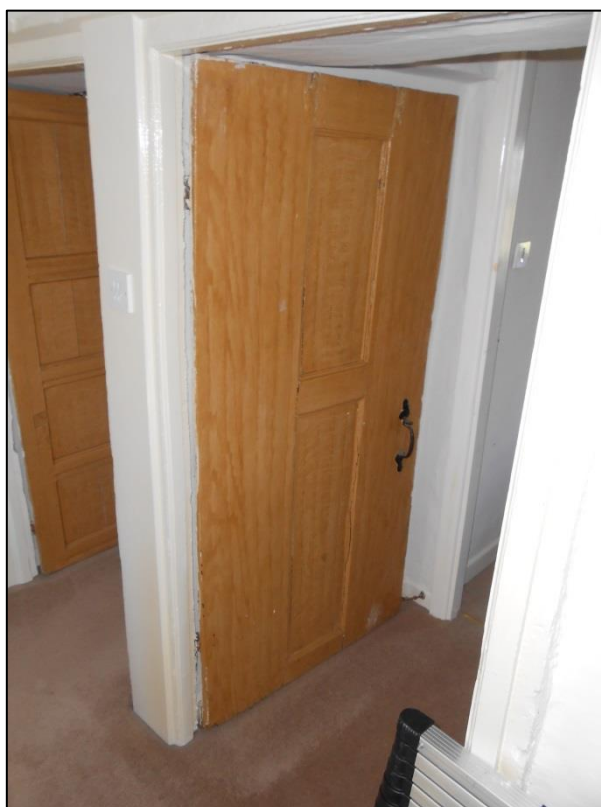
PL00: Original internal door present to the first floor of the building to the front north west bedroom
