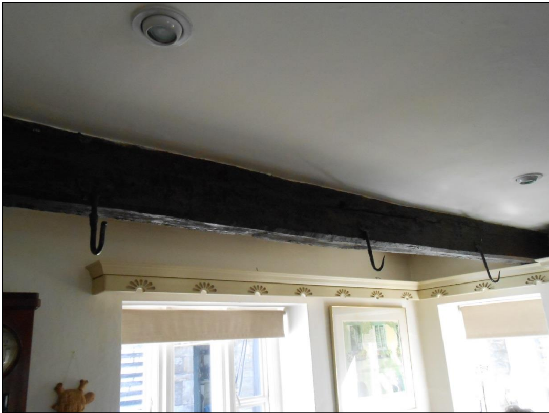
PL00: Hooks present to the underside of a timber beam to the kitchen ceiling.
