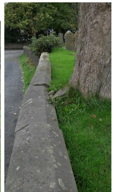
Detail showing displaced copings
