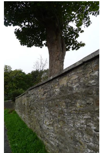
Bellying stone wall, adjacent to roadway
