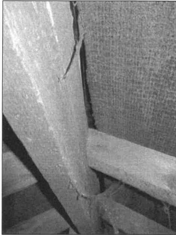
Plate 11: In the southern aspect of the house, there was a substantial gap between the roofing membrane and the ridge beam, sufficient for bats to use.
