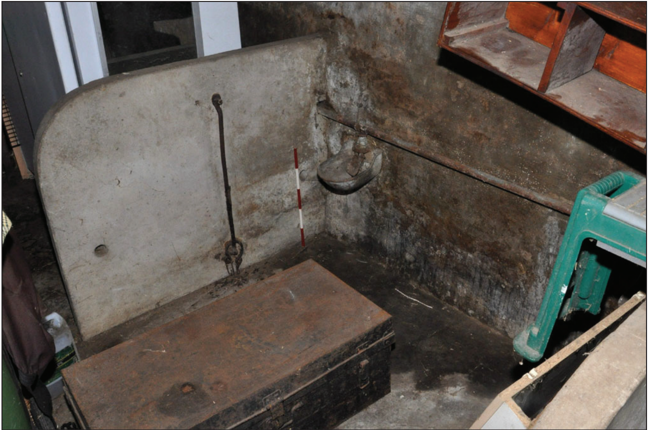
Photo 27: Concrete boskin and floor in north-east shippon
