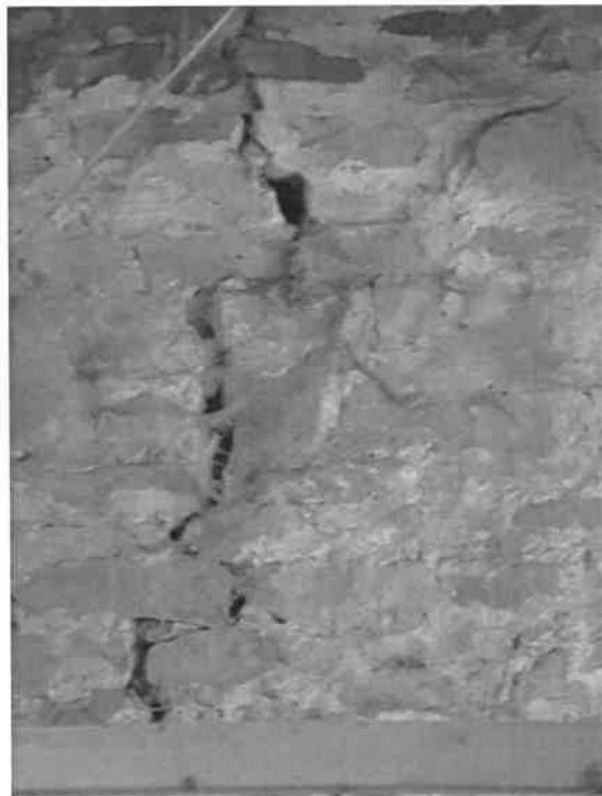
CRACK TO SIDE OF STAIR
