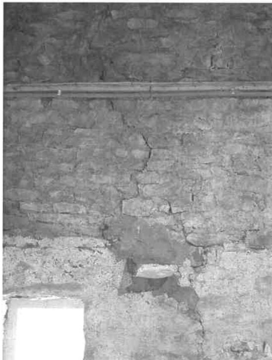
CRACKING TO INTERNAL FACE OF LEFT HAND WALL
