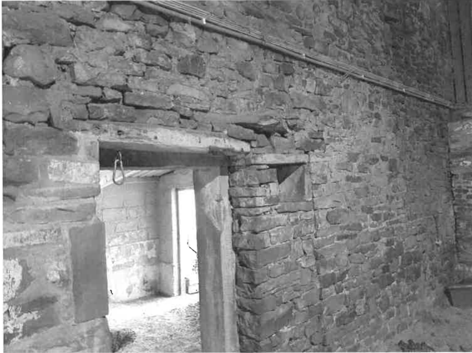
DISTURBANCE OF STONework OVER OPENING TO EXTENSION
