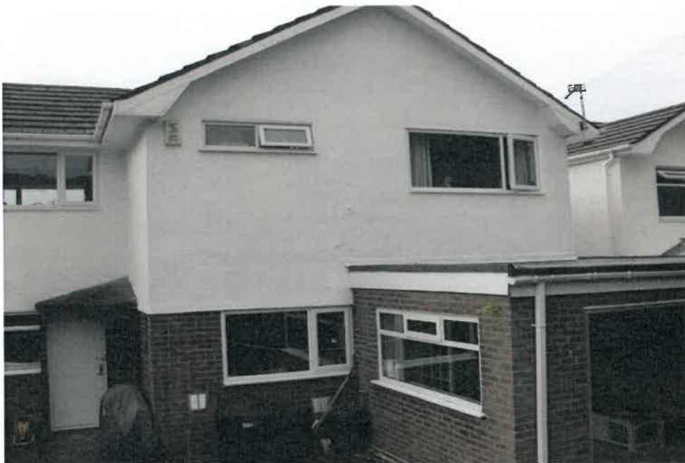
Rear of House showing the connection of the Garden Room to the House
