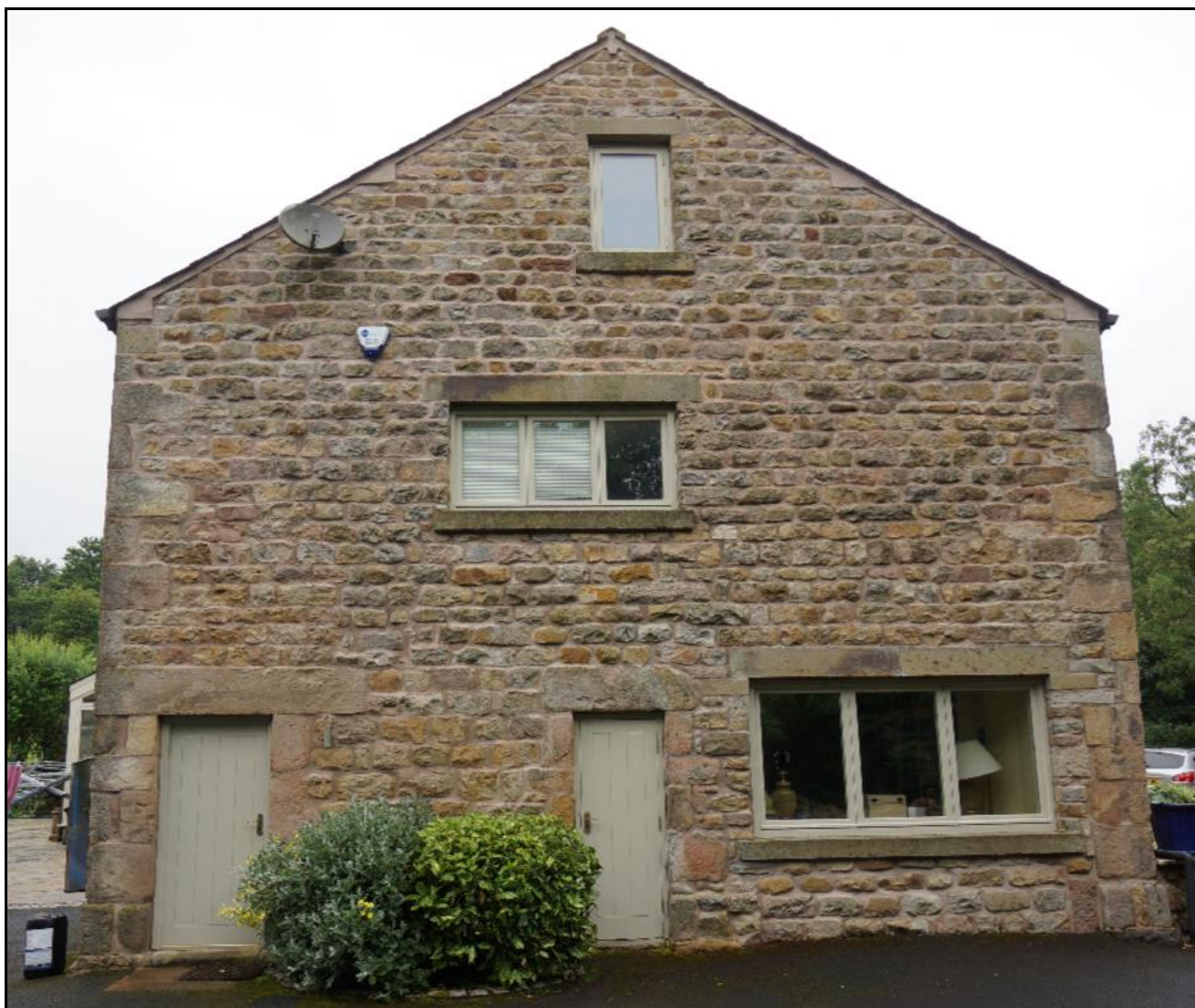
Figure 9) Southern elevation with raised gable, inserted right hand window and inserted windows above. The central and left hand doors appear to be original shippon doors
