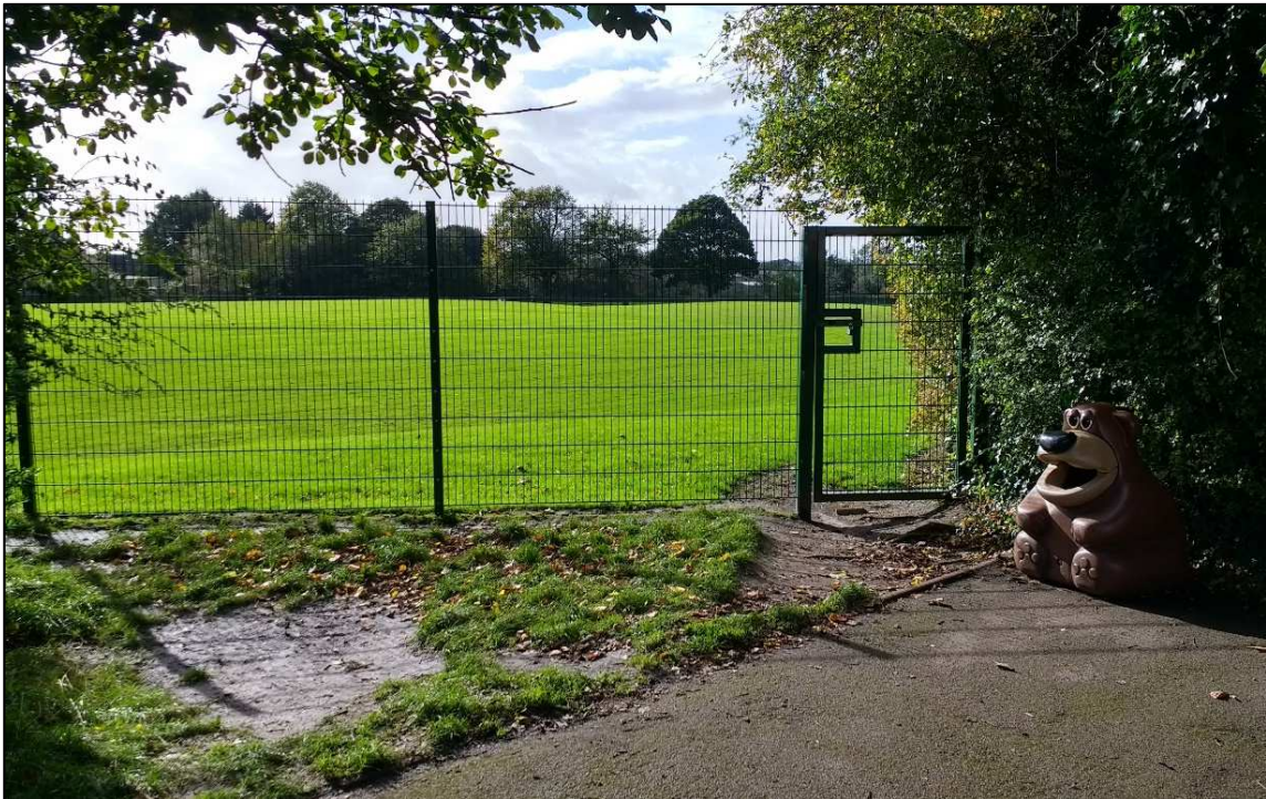
Figure 3: Existing Rear Fence at the Southern Boundary
