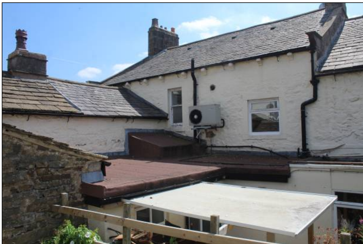
8. Clutter of modern lean-to structures at the rear masks the ground floor
