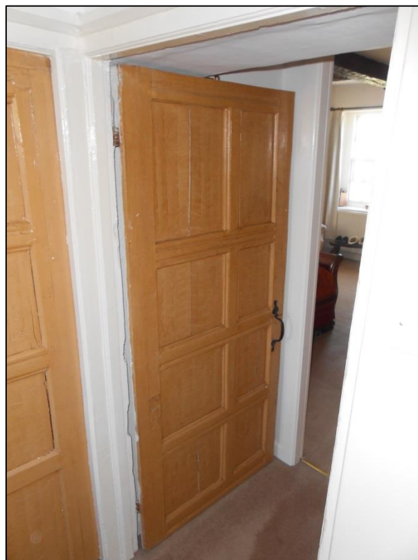
PL00: Original internal door present to the first floor of the building to the front south west bedroom
