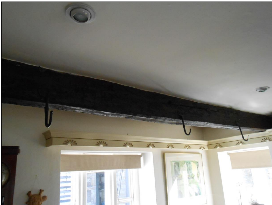
PL00: Hooks present to the underside of a timber beam to the kitchen ceiling.
