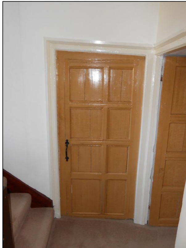
PL00: Original internal door present to the first floor of the building (now fixed shut) to the south east of the building.
