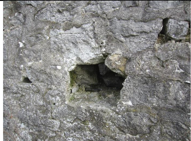
Photo 2: Gaps in the stone work
