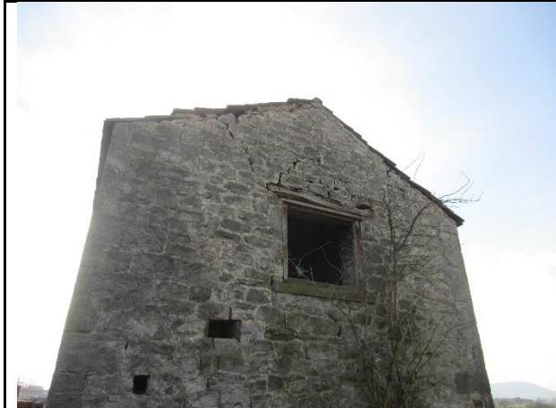
Photo 1: North elevation of stone barn showing gaps in the stonework and beneath the window lintel
