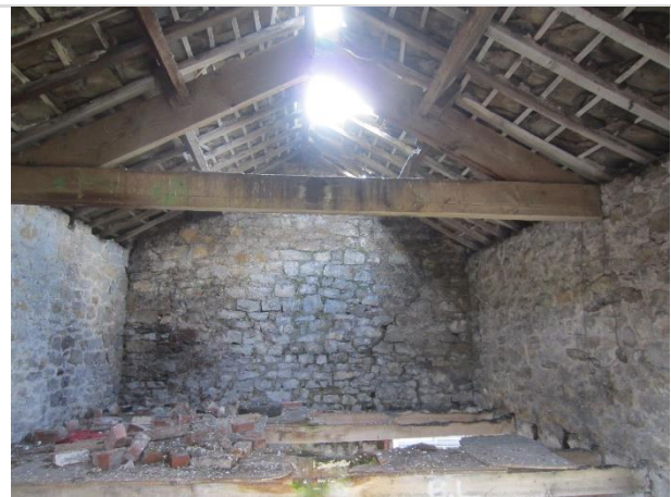
Photo 4: Interior of stone barn showing mortared / pointed internal walls and feral pigeon droppings
