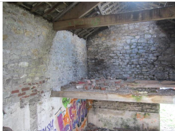
Photo 3: Interior of stone section showing dilapidated timber hayloft
