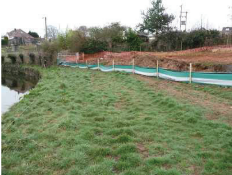
Example of installation of silt fencing, and attached example of manufacturers detail
