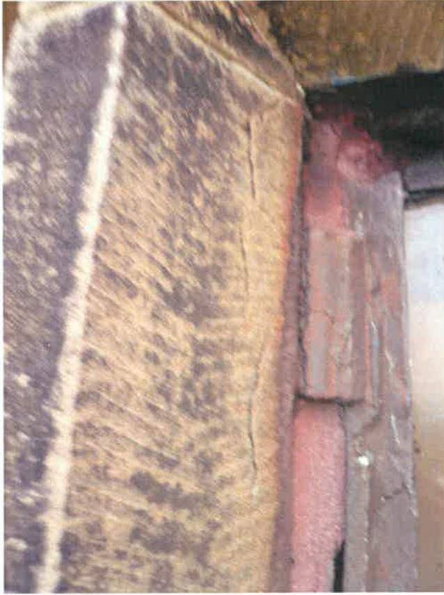
Image 2 shows further cracks on the left hand section of the mullion.
