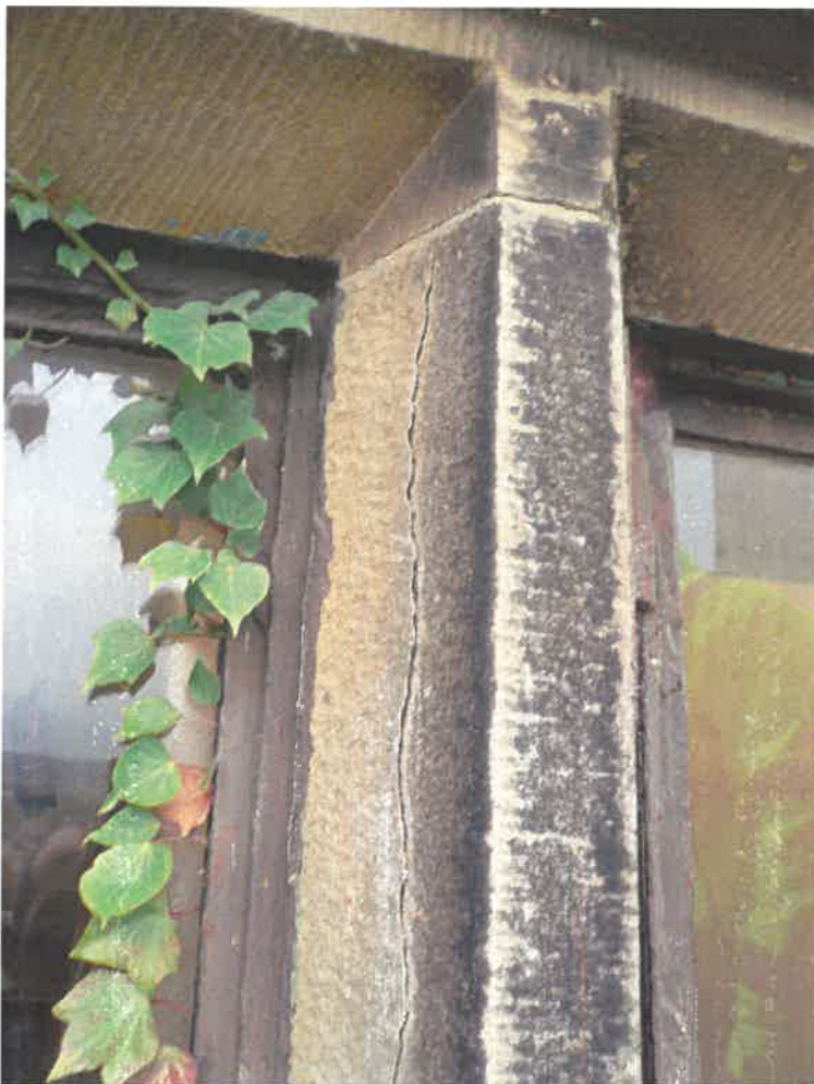
Image 1. Vertical cracking to the central mullion.
