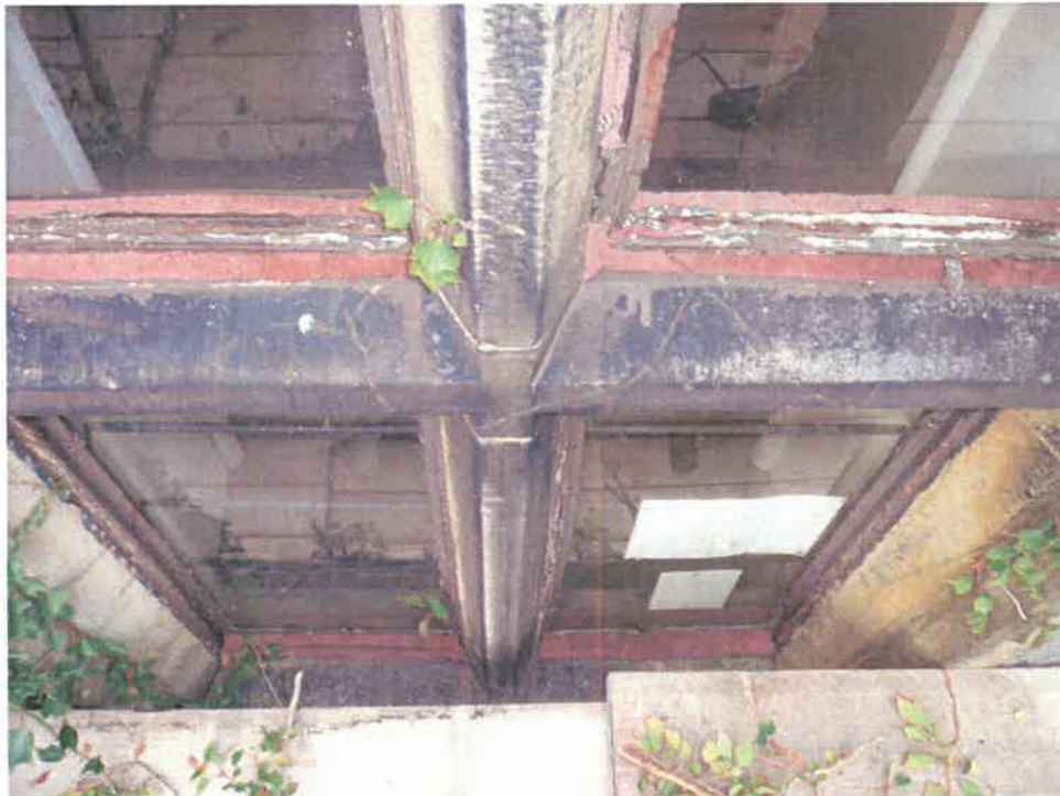
Image 3 Evidence of previous repair to the lower section of the mullion.
