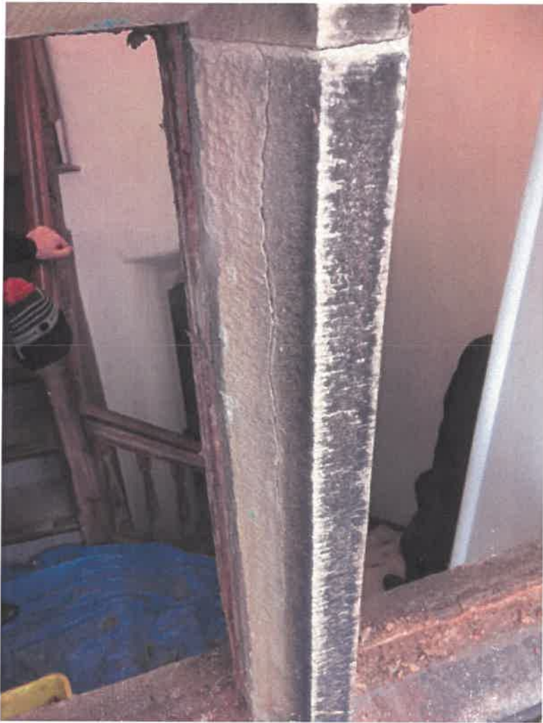
Image 4 Crack on Mullion once the window frames were removed.
