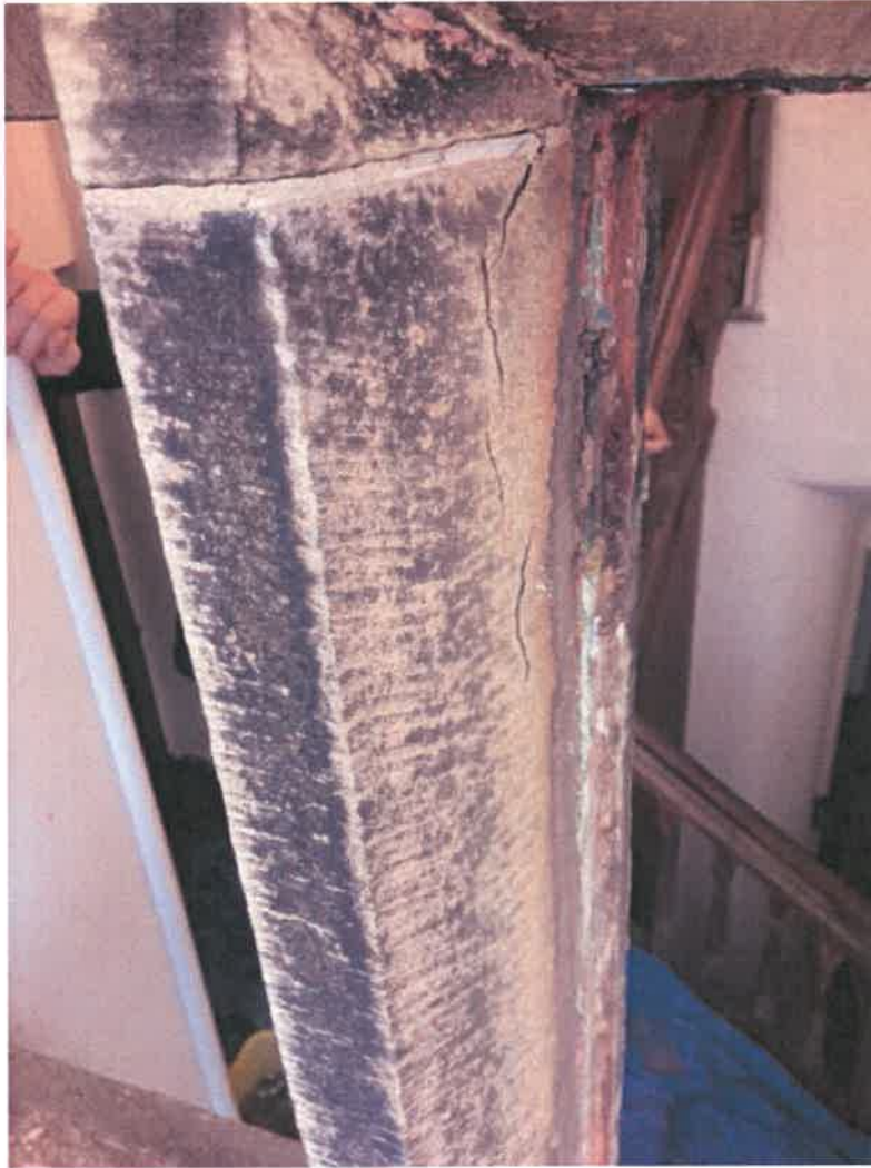
Image 5 crack on the left hand side once the window frames were removed.
