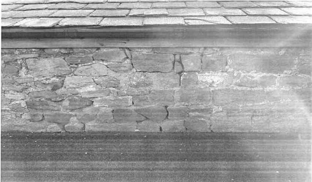
Photograph 4: Example of the gaps and cracks in the stone work on the northern façade
