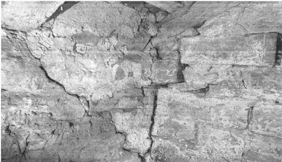
Photograph 12: Example of cracks and gaps in the stonework of rooms B, C, and D.
