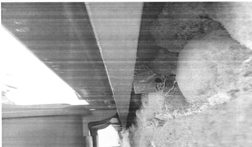
Photograph 7: An example of gap behind the bargeboard.
