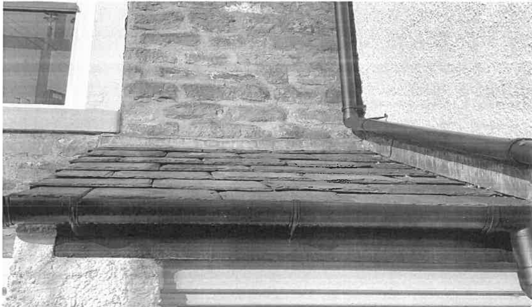
Photograph 14: Example of natural lifting of the roof slates above the entrance porch.
