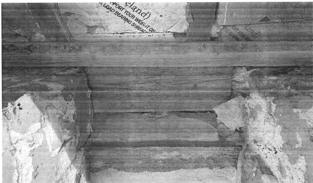
Photograph 10: Gaps around wooden lintel in the window.
