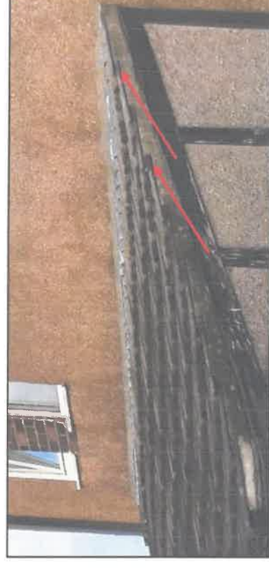
Photo 5: B1, front (south) elevation, showing the gaps in the roof tiles at the leading edge.
