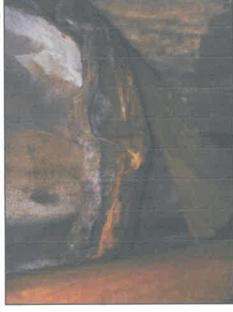
Photo 7: Close up of broken roof timber and felt, exposing the underside of roof tiles.
