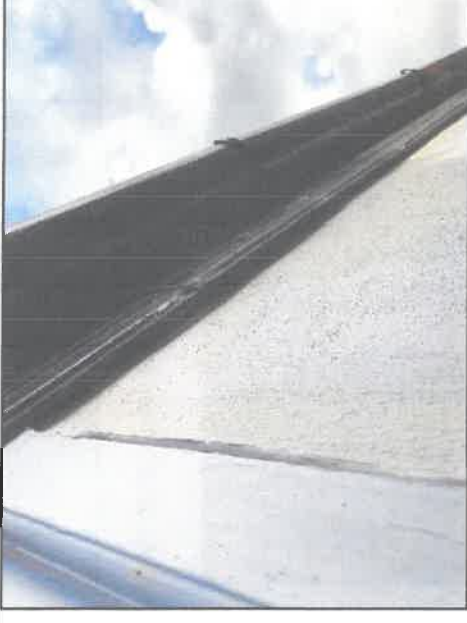
Photo 4: Showing the gap behind the barge board on the west elevation of the lean-to.
